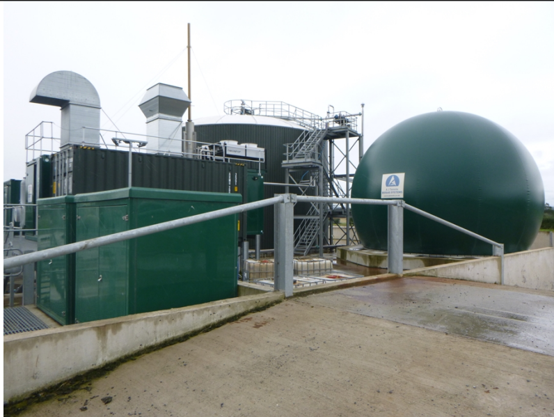
Image 3: Infrastructure within the AD Plant bund
