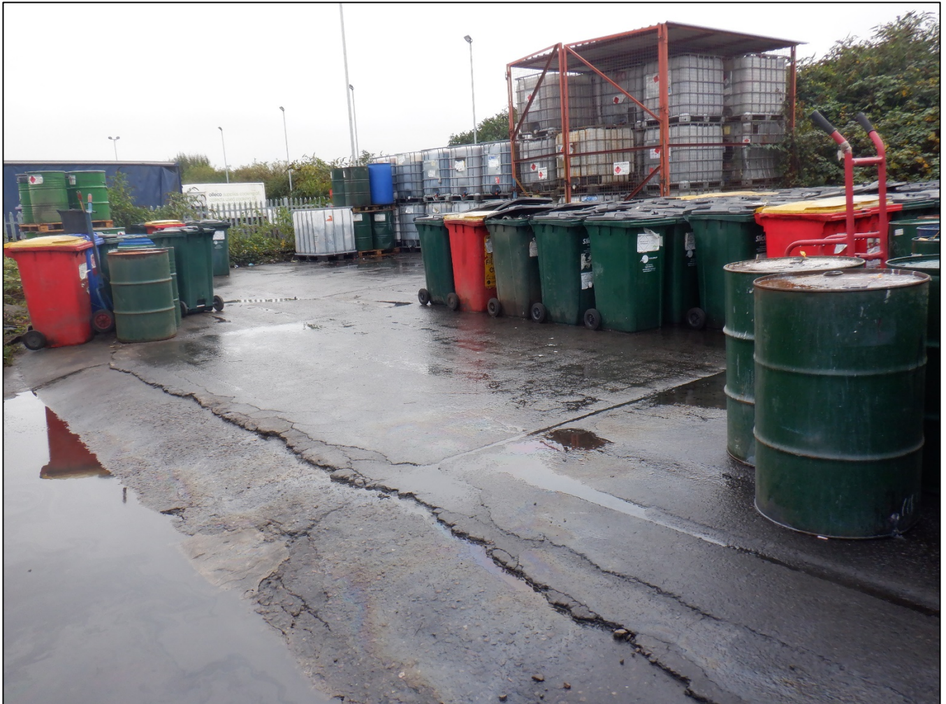
Photograph 1. Waste storage area. Damaged concrete, standing water, evidence of oil spill/leak and surface profile causing (contaminated) surface waters to flow away from drainage infrastructure.
