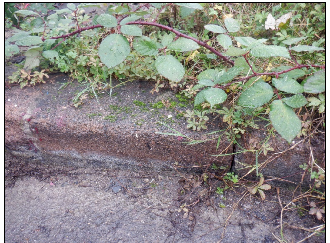
Photograph 3. Waste storage area. Damaged concrete lip.
