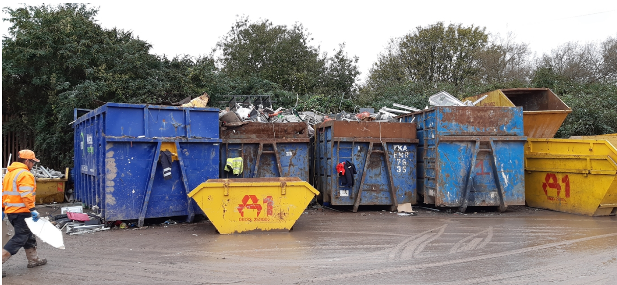
Photo 1 - General condition of on site housekeeping
