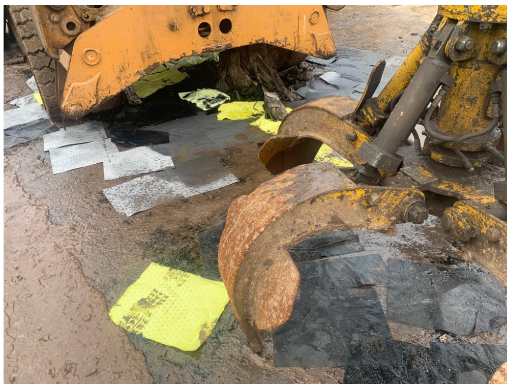
Photo 3 - Oil remediation measures in place following our site visit (Photo taken and provided by Site Manager Mr. Chris JONES following our site visit on 09/11/21)
