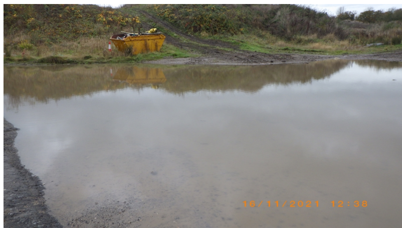
Photo showing large pool of standing water
