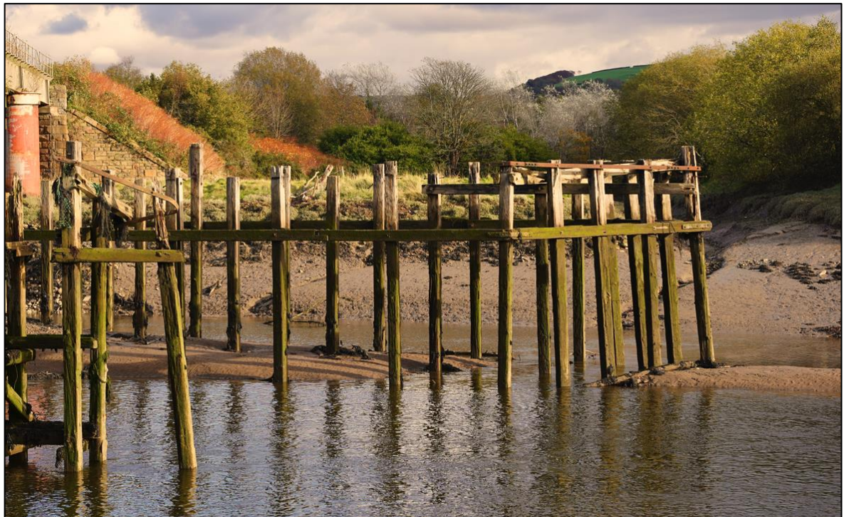
Figure 3: Timber Pontoon to be removed as part of the works, as this is redundant and in danger of collapse.
