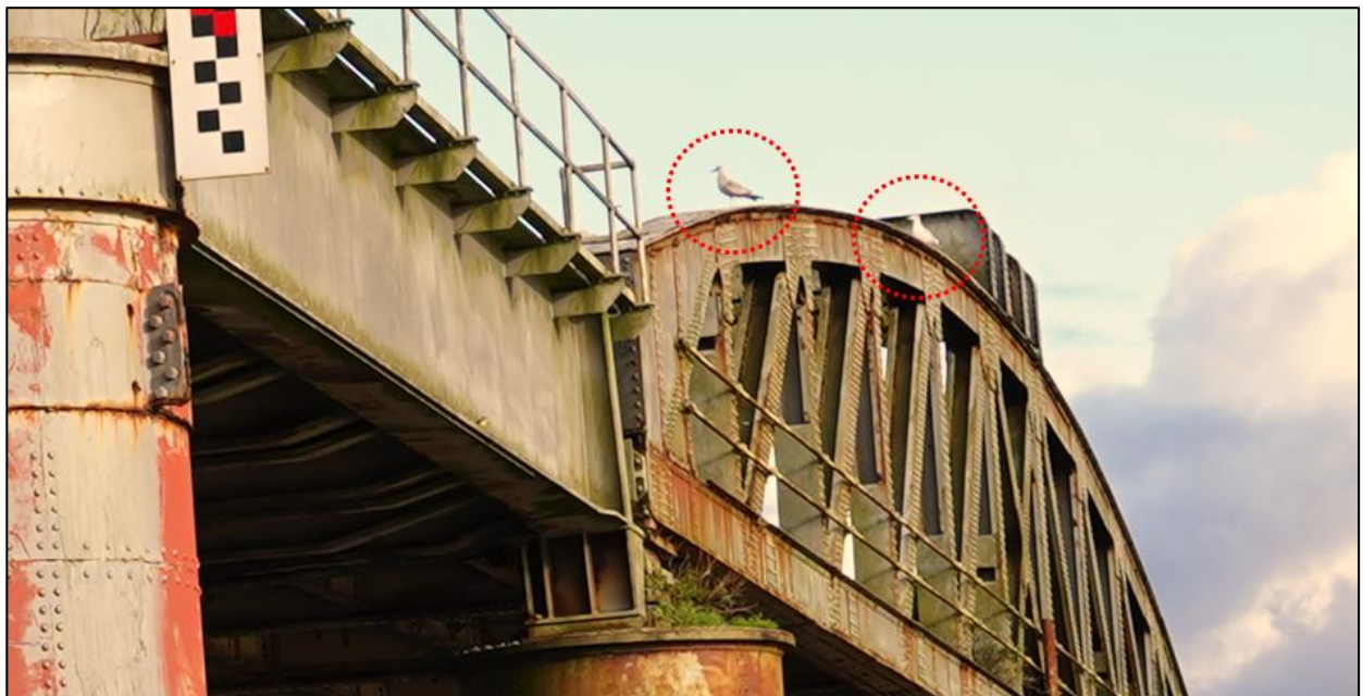
Figure 11: Gul observed perching on steelwork.
