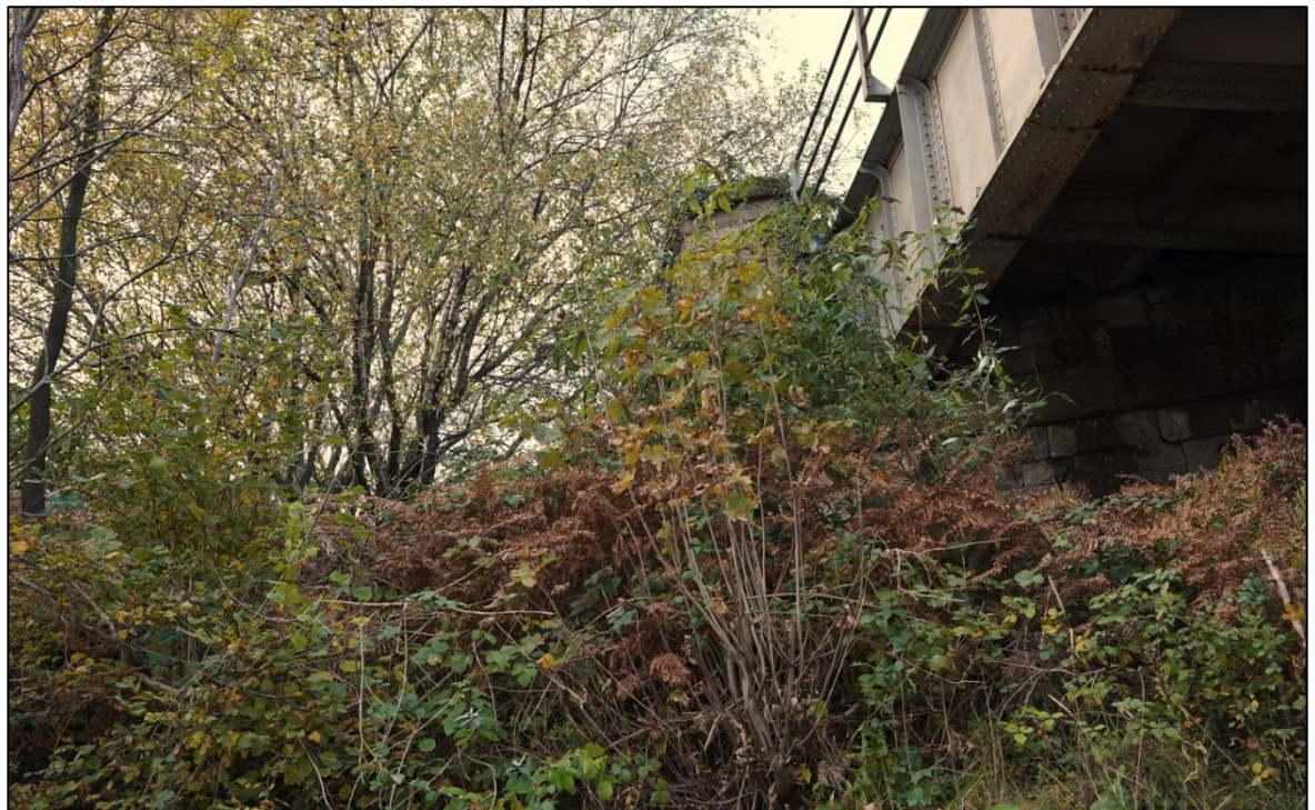
Figure 8: Mixed dense vegetation below and adjacent to southwest masonry abutment.
