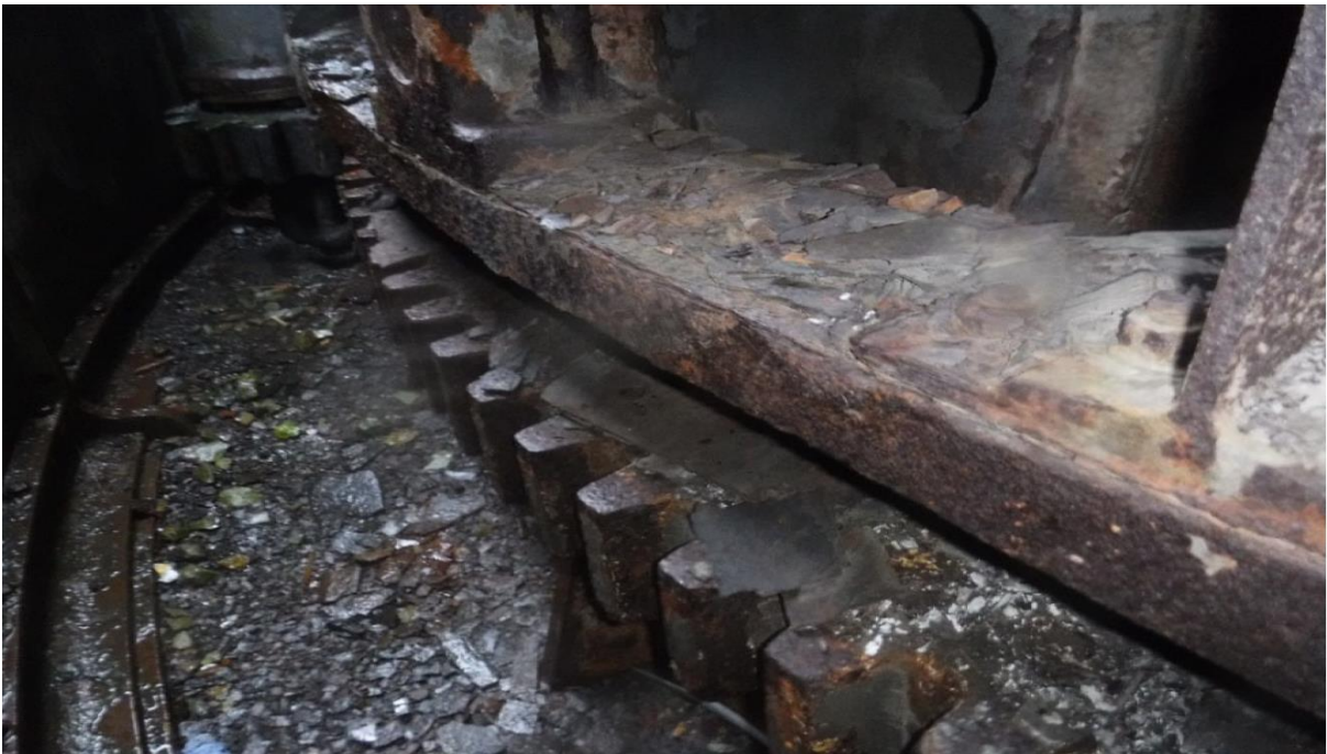
Figure 15: Internal gearing of Swing Bridge.
