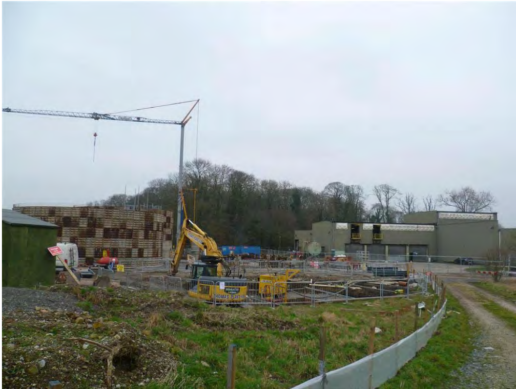
Photograph 3: Location of SAS buffer tank, thickener feed pumps and mixer
