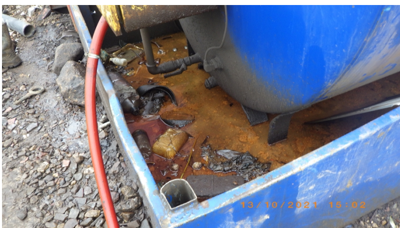
Photos showing fuel tank and bund
