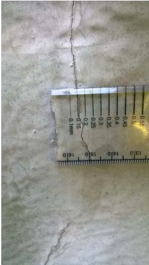
Photo 4.3.1: Truefloc TAc40 – Crack in concrete block masonry wall
