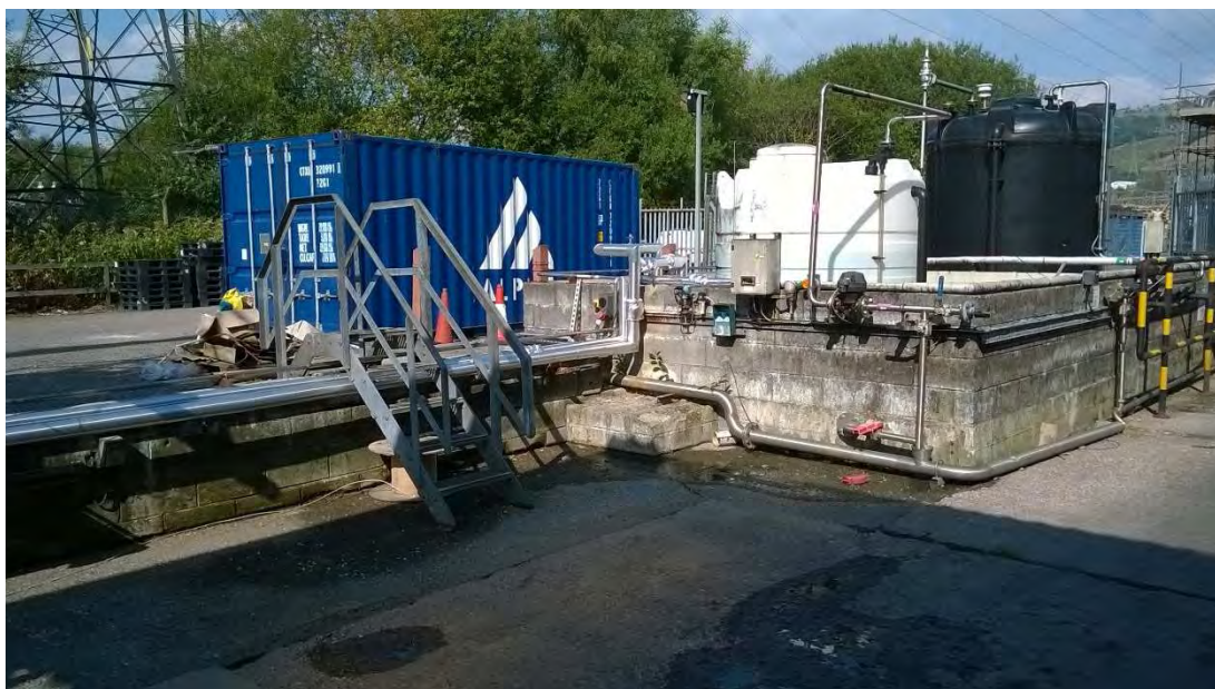
Figure 4.9.1: Photograph of Acetic Acid tank (white) and Bund
