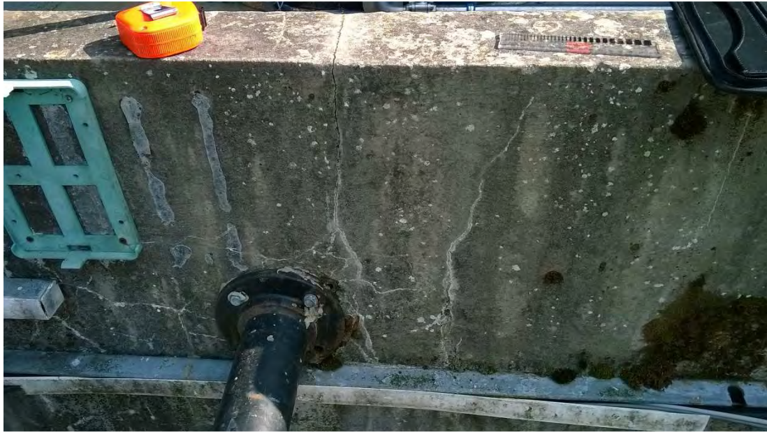
Photo 4.10.2: Phosphoric Acid – Crack in concrete block masonry wall (2)
