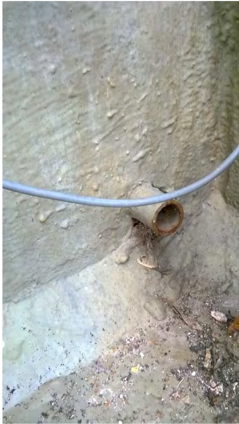
Photo 4.3.3 : Truefloc TAC40 – Unsealed Penetration through bund wall
