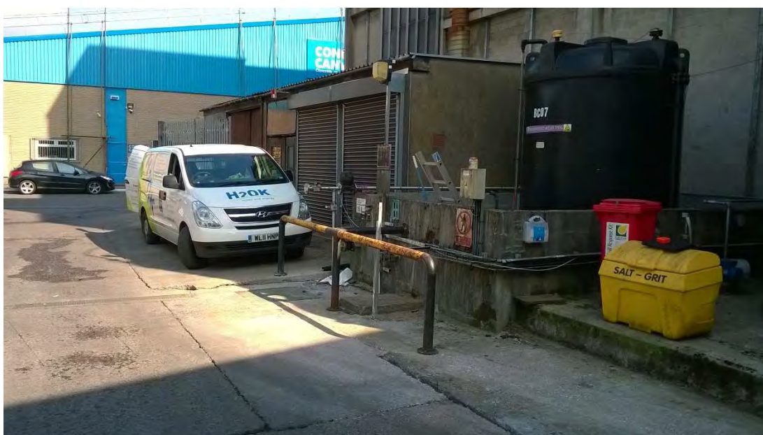
Figure 4.10.1: Photograph of A21 Phosphoric Acid Tank and Concrete Block Masonry Bund
