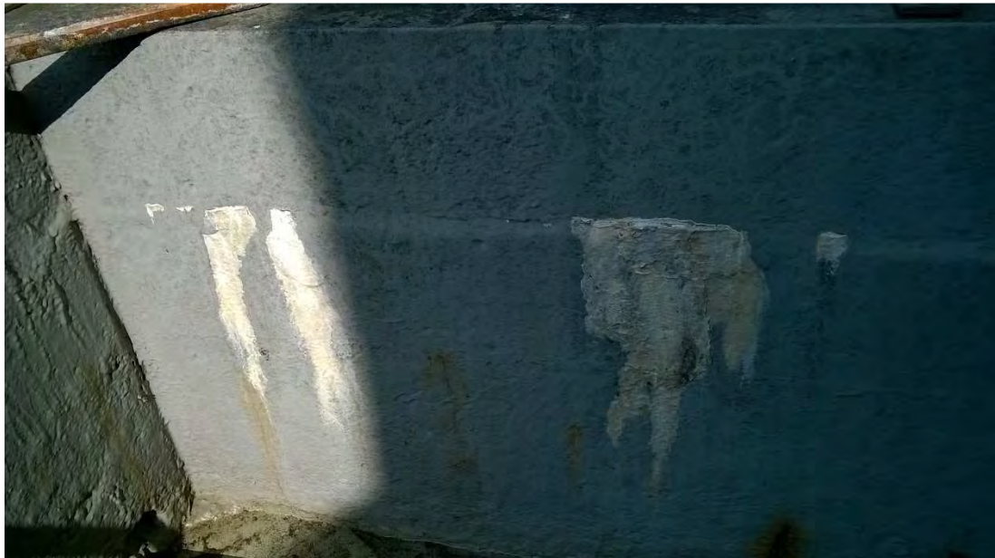
Photo 4.10.3: Phosphoric Acid – Crack in concrete block masonry wall (3)
