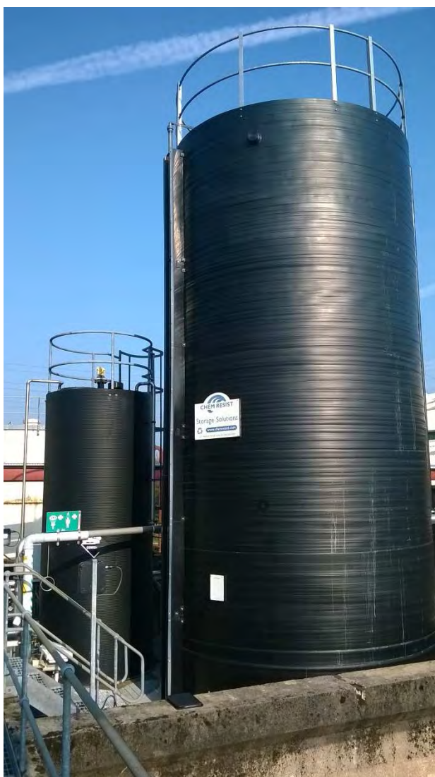
Figure 4.5.1: Photograph of Caustic Day Tank Primary Vessel (left) and Caustic Tank (right) on Suspended Steelwork Floor above Reinforced Concrete Bund
