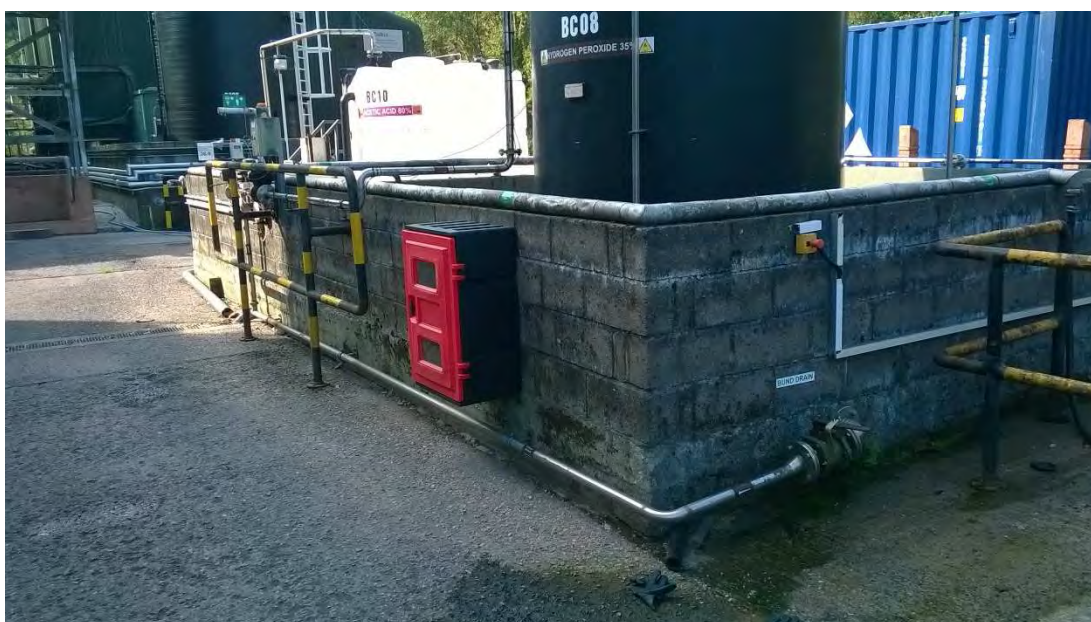
Figure 4.8.1: Photograph of Hydrogen Peroxide tank (black) and Bund
