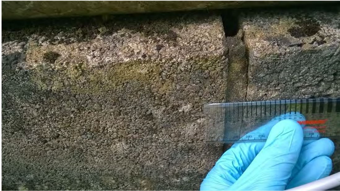
Photo 4.8.2: Hydrogen Peroxide – Crack in concrete block masonry wall (2)
