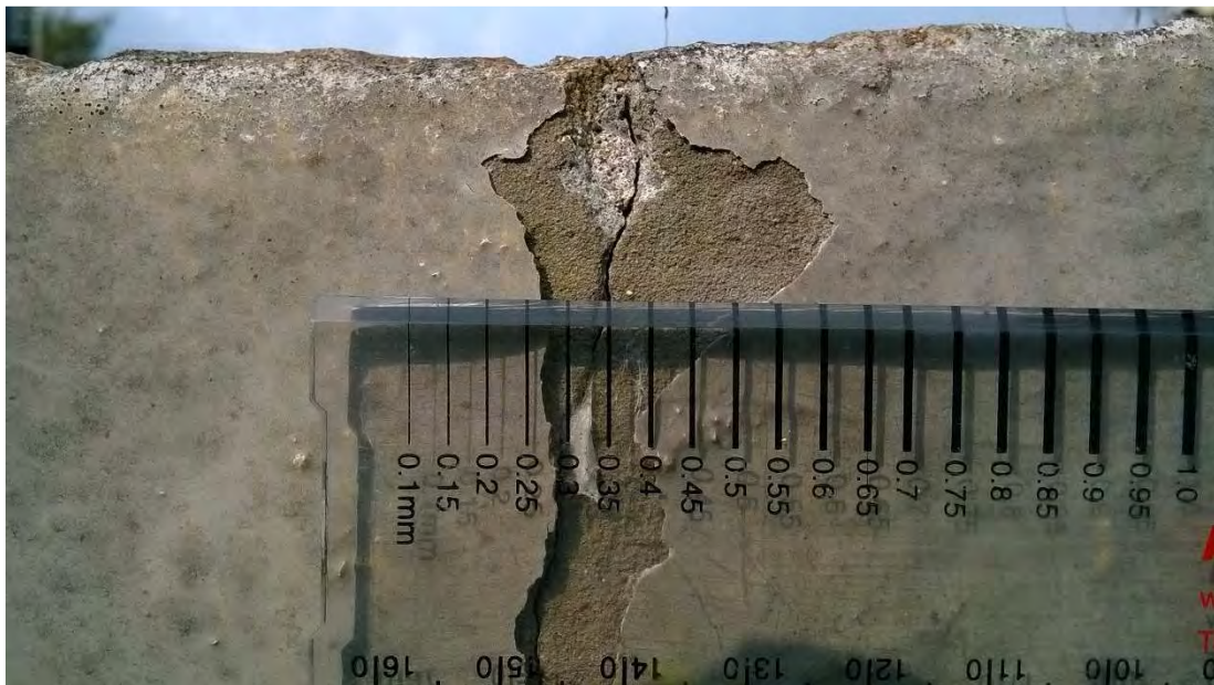
Photo 4.3.2: Truefloc TAc40 – Crack in concrete block masonry wall
