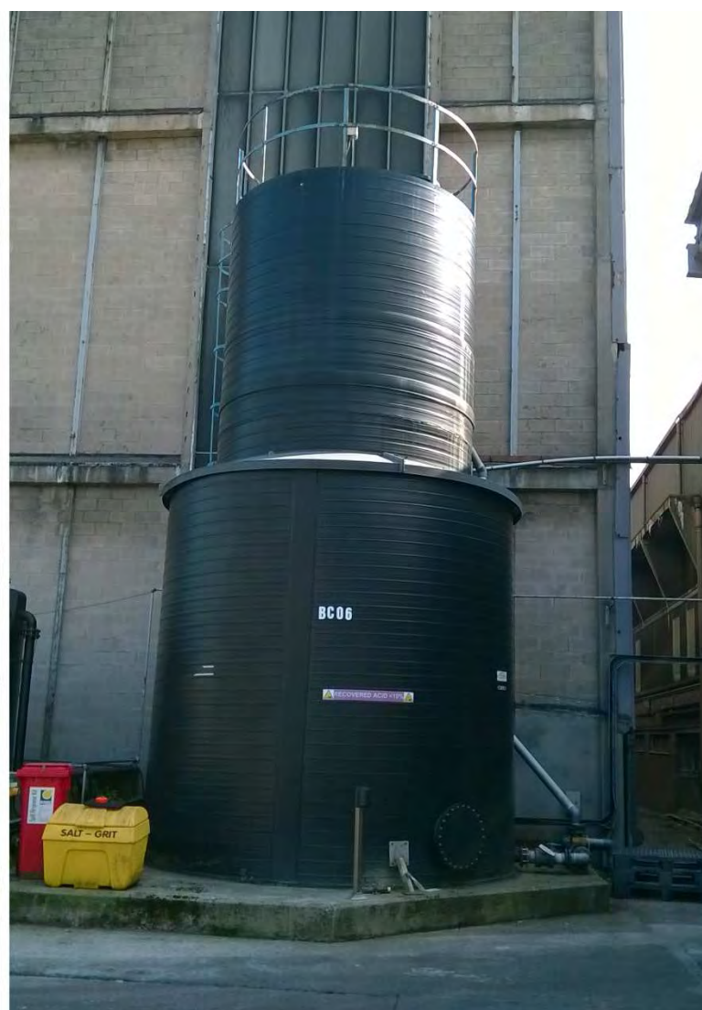
Figure 4.6.1: Photograph of A21 Deioniser Effluent (Diluted HCL) Primary Tank with Collar Bund
