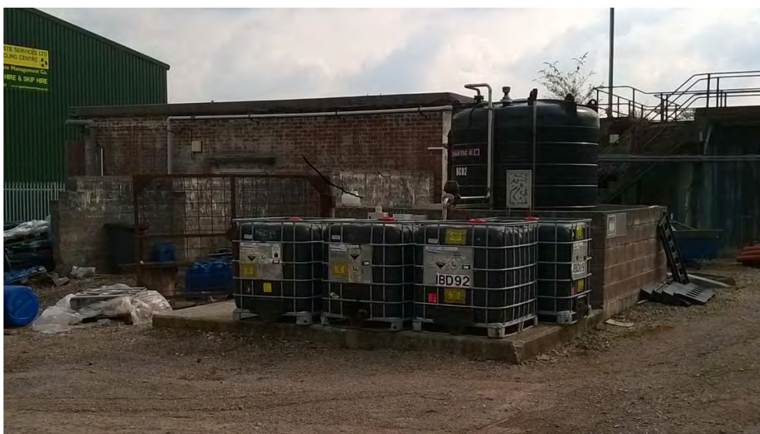
Figure 4.3.1: Photograph of Truefloc TAC40 Primary Tank within Block Masonry Bund
