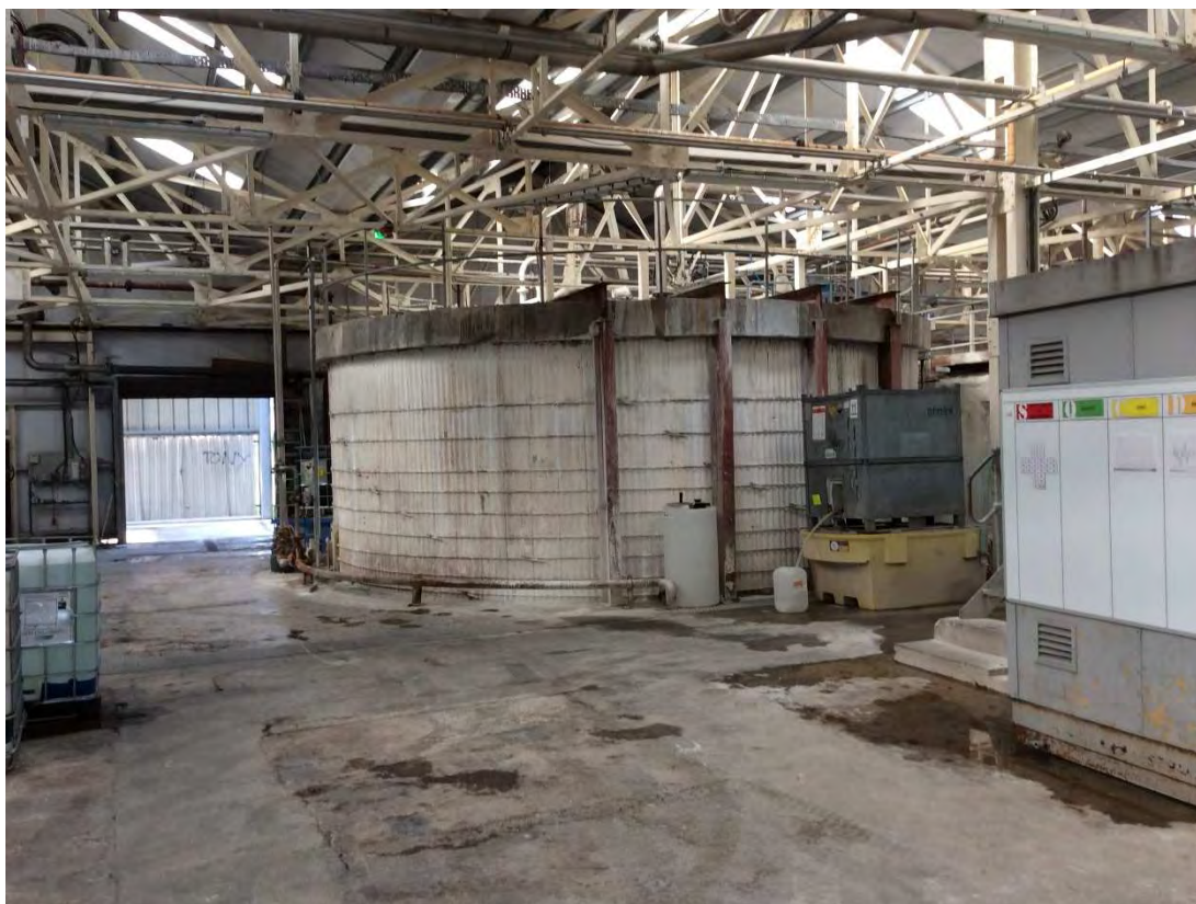
Figure 4.11.1: Photograph of A18 Hydrated lime Primary Tank
