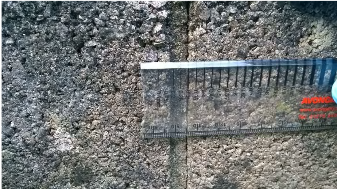
Photo 4.9.2: Acetic Acid – Crack in concrete block masonry wall (1)
