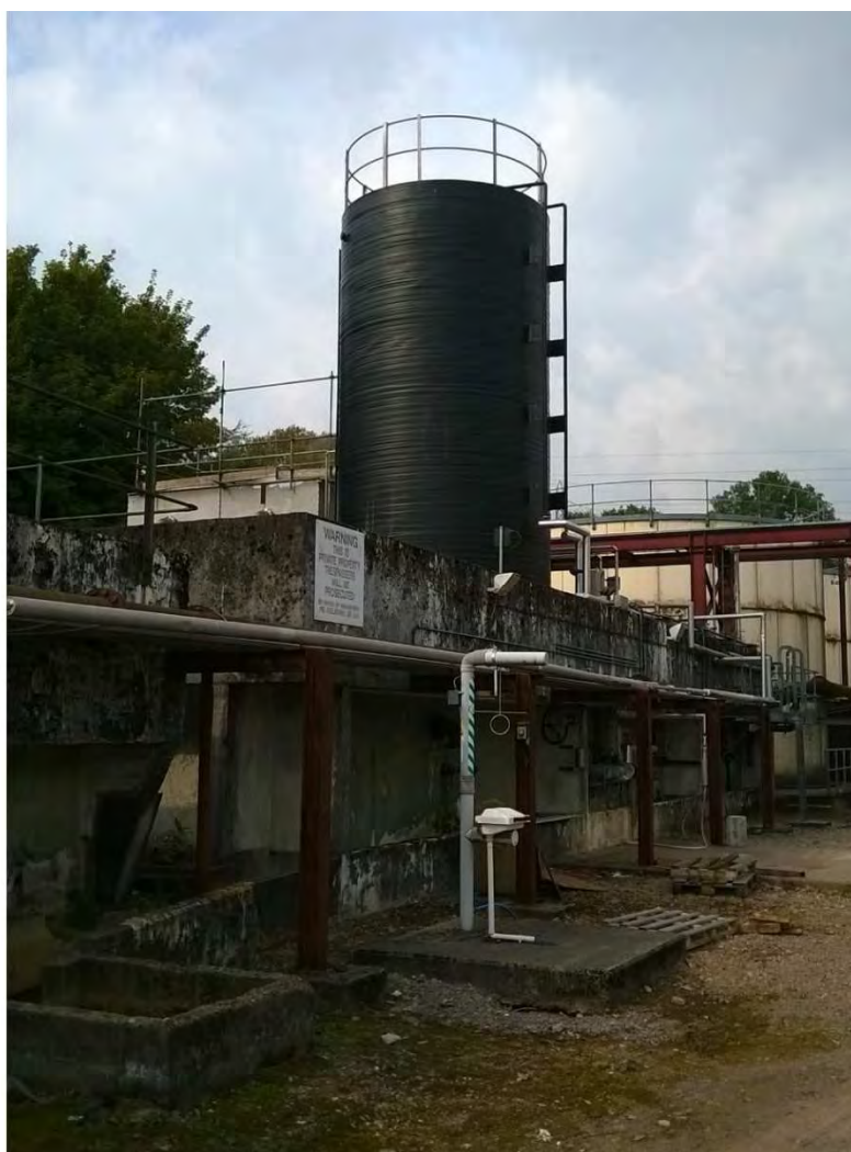
Figure 4.4.1: Photograph of Caustic Primary Tank within Reinforced Concrete Bund
