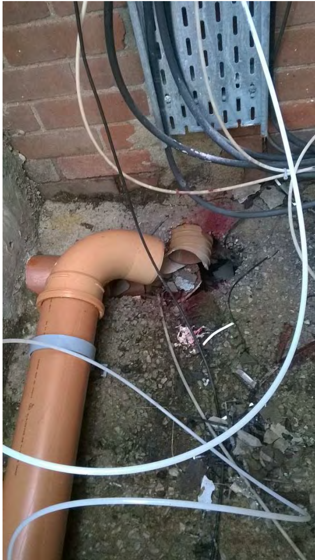
Photo 4.7.1: Hydrochloric Acid Tank Tertiary Containment Drainage – Damaged/missing section of drainage
