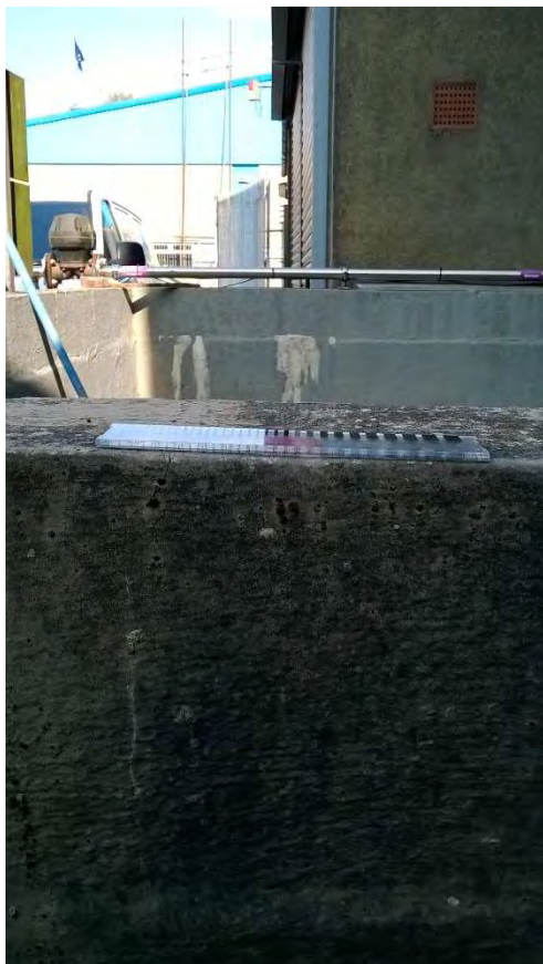
Photo 4.10.1: Phosphoric Acid – Crack in concrete block masonry wall (1)
