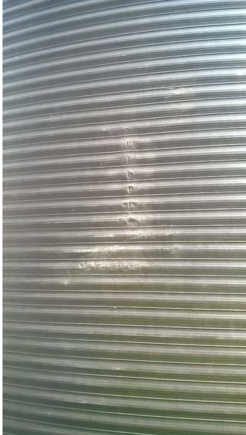
Photo 4.5.2: Caustic Day Tank – Damage to tank wall (2)
