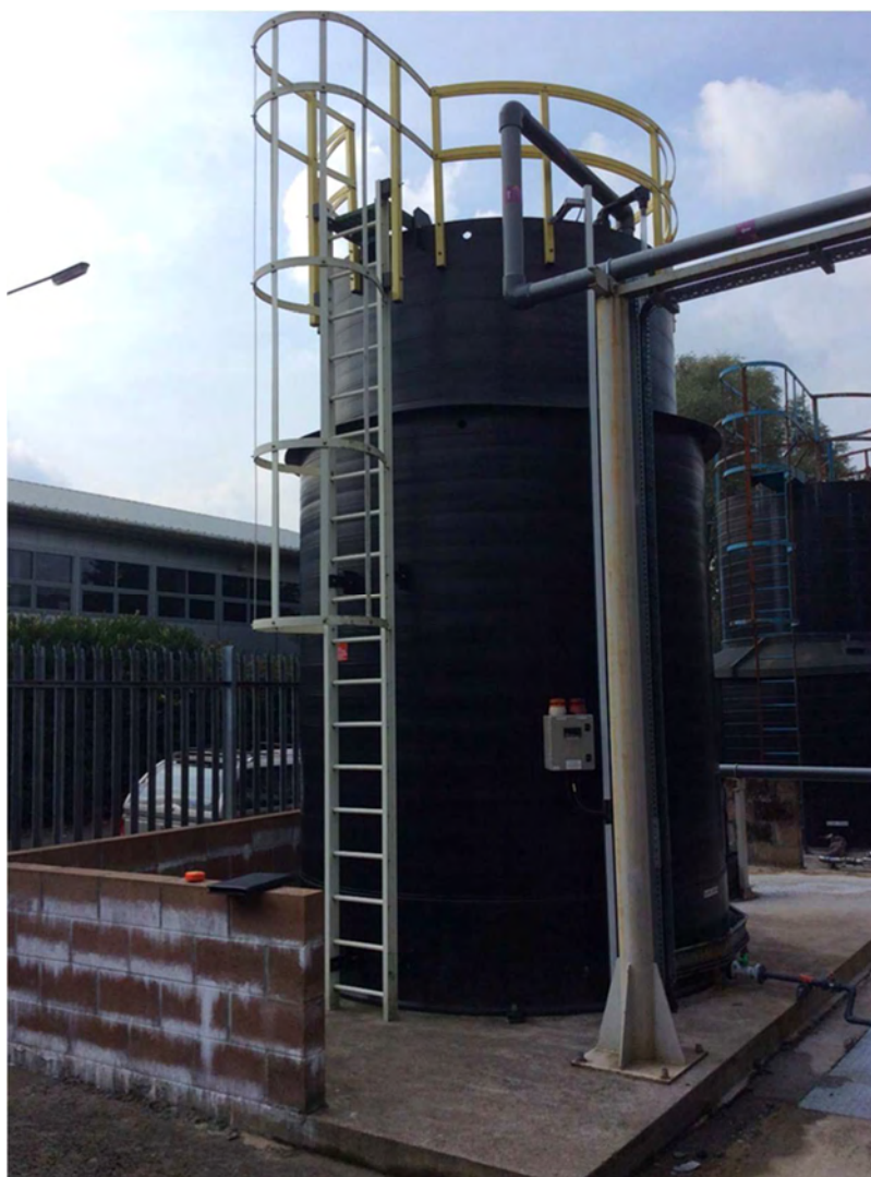
Figure 4.2.1: Photograph of A18 Sulphuric Primary Tank with Collar Bund
