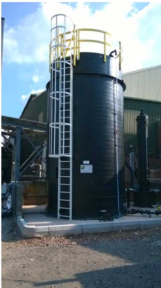
Figure 4.7.1: Photograph of A21 Hydrochloric Acid Primary Tank with Collar Bund
