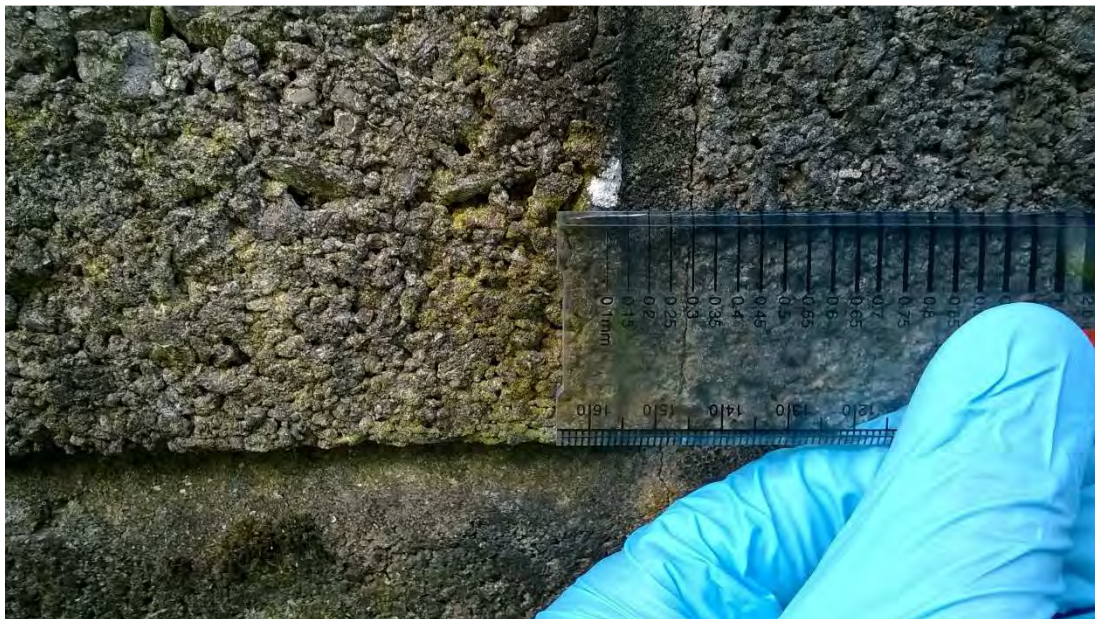
Photo 4.8.1: Hydrogen Peroxide – Crack in concrete block masonry wall (1)
