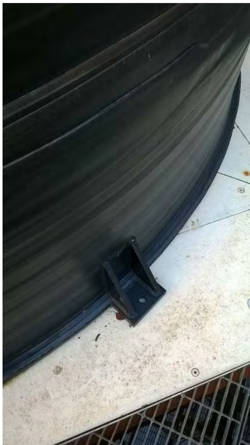
Photo 4.4.1 : Caustic Tank – Holding down bolts missing at base of tank
