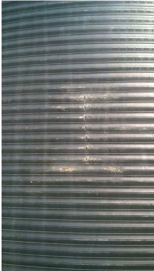
Photo 4.5.3 : Caustic Day Tank – Damage to tank wall (3)
