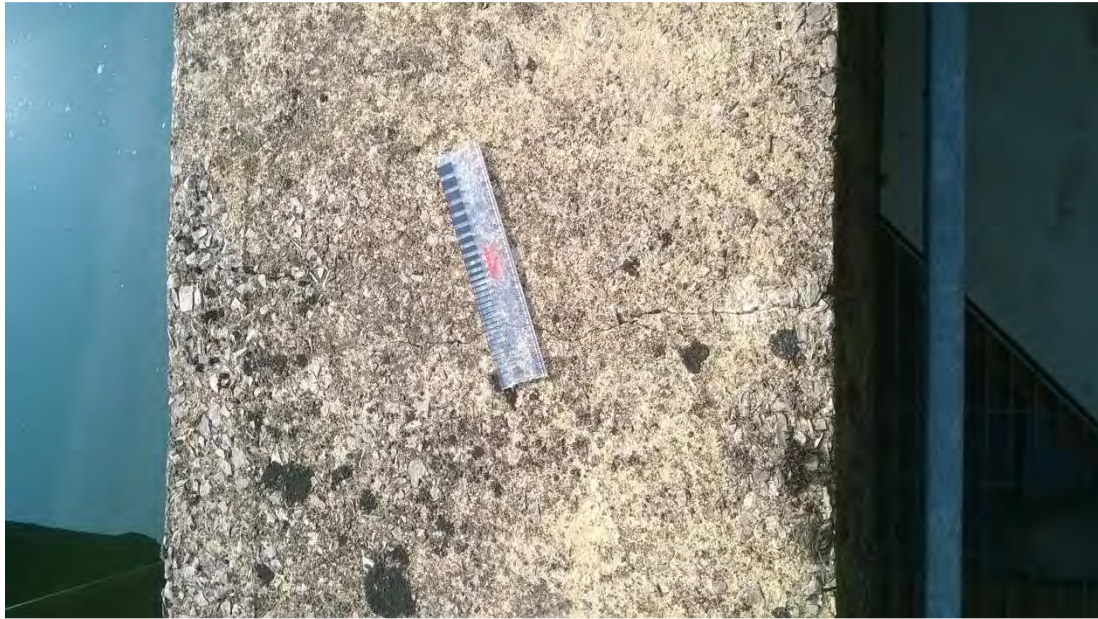
Photo 4.4.2 : Caustic Tank – Crack through wall (1) viewed from above
