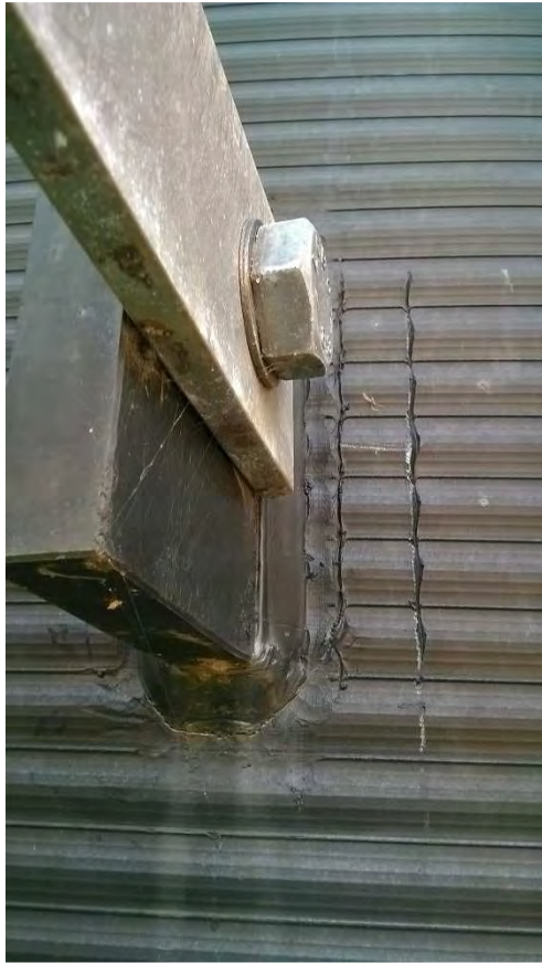
Photo 4.5.1: Caustic Day Tank – Damage to tank wall (1)
