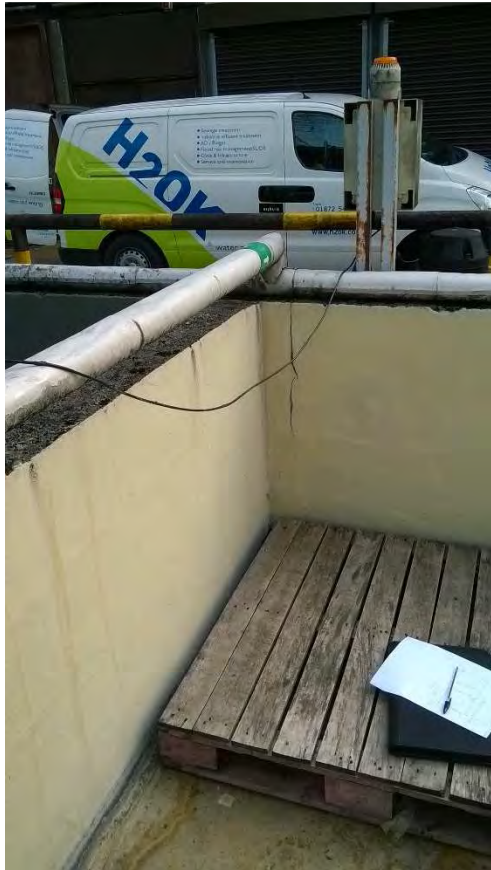
Photo 4.9.4: Acetic Acid – Crack in concrete block masonry wall (3)
