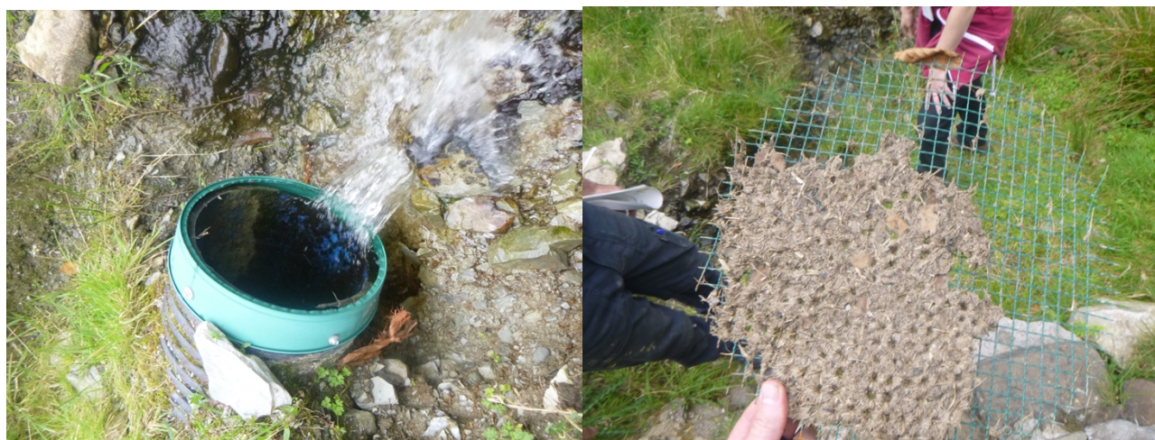
Figures 4 & 5: Discharge Outlet pipe and Screen
