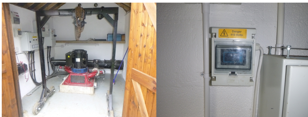
Figure 2 & 3: The turbine and meter
