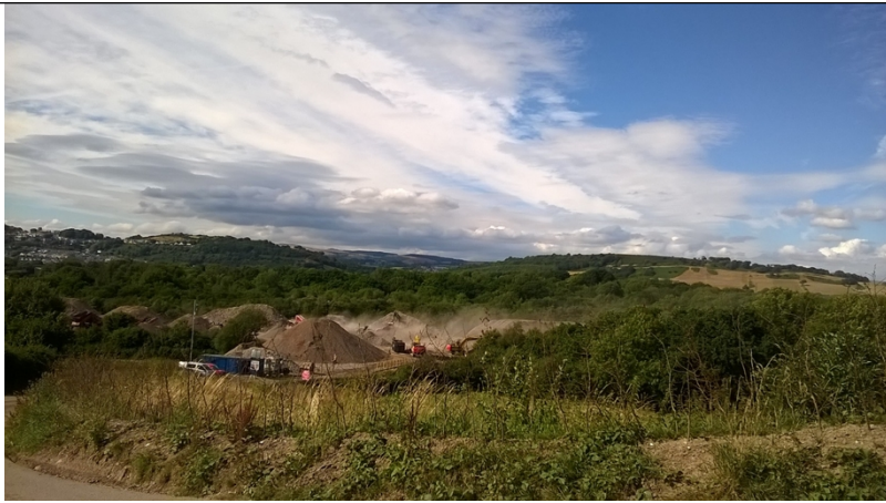
Dust seen coming from the crusher.
