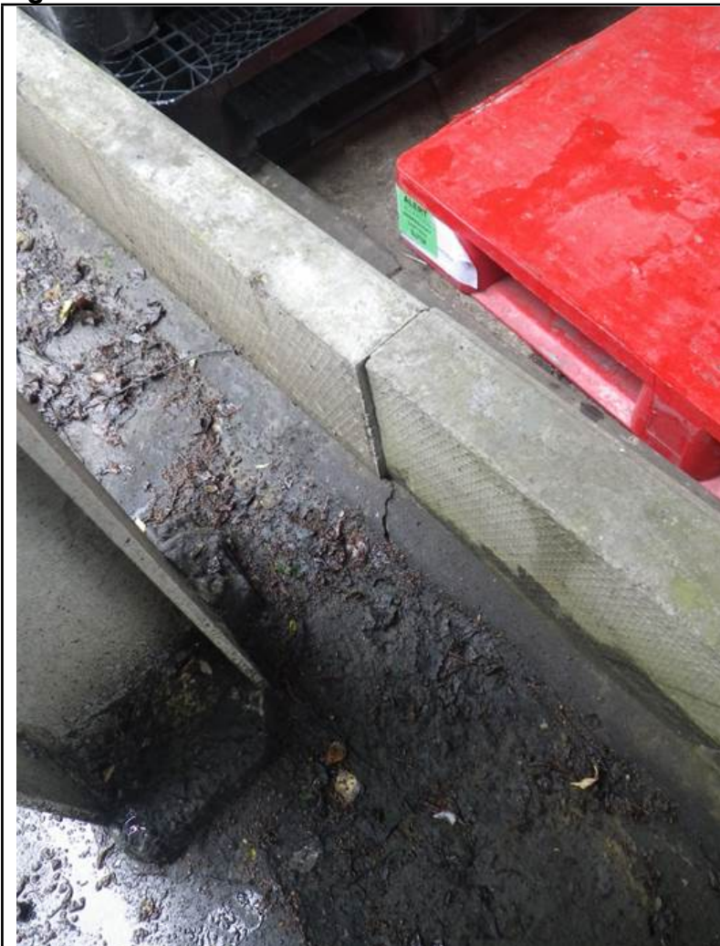
Figure 2: Cracks in bund
