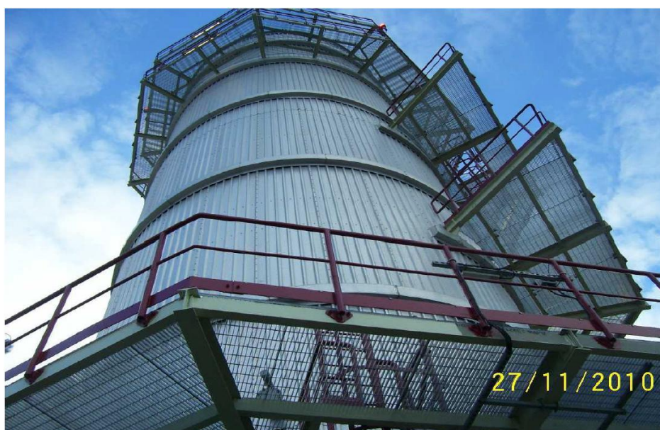
Figure 1 Typical exhaust stack and sampling platform
