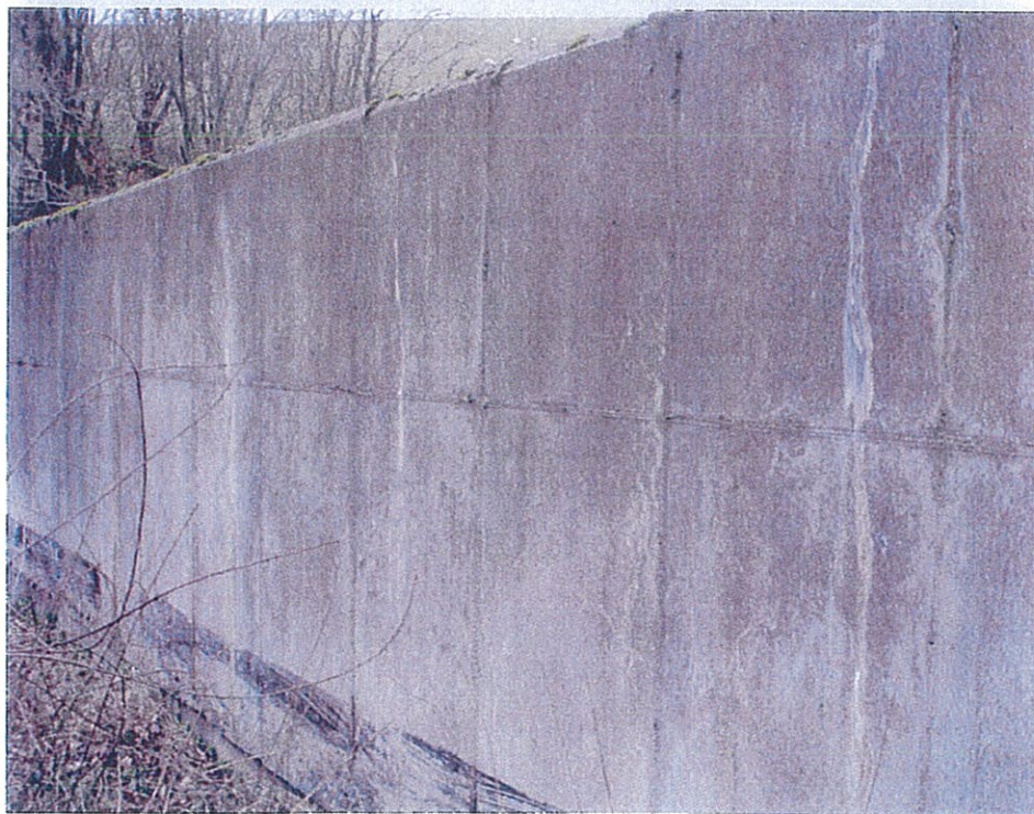
Photograph 5: South wall – typical cracking
