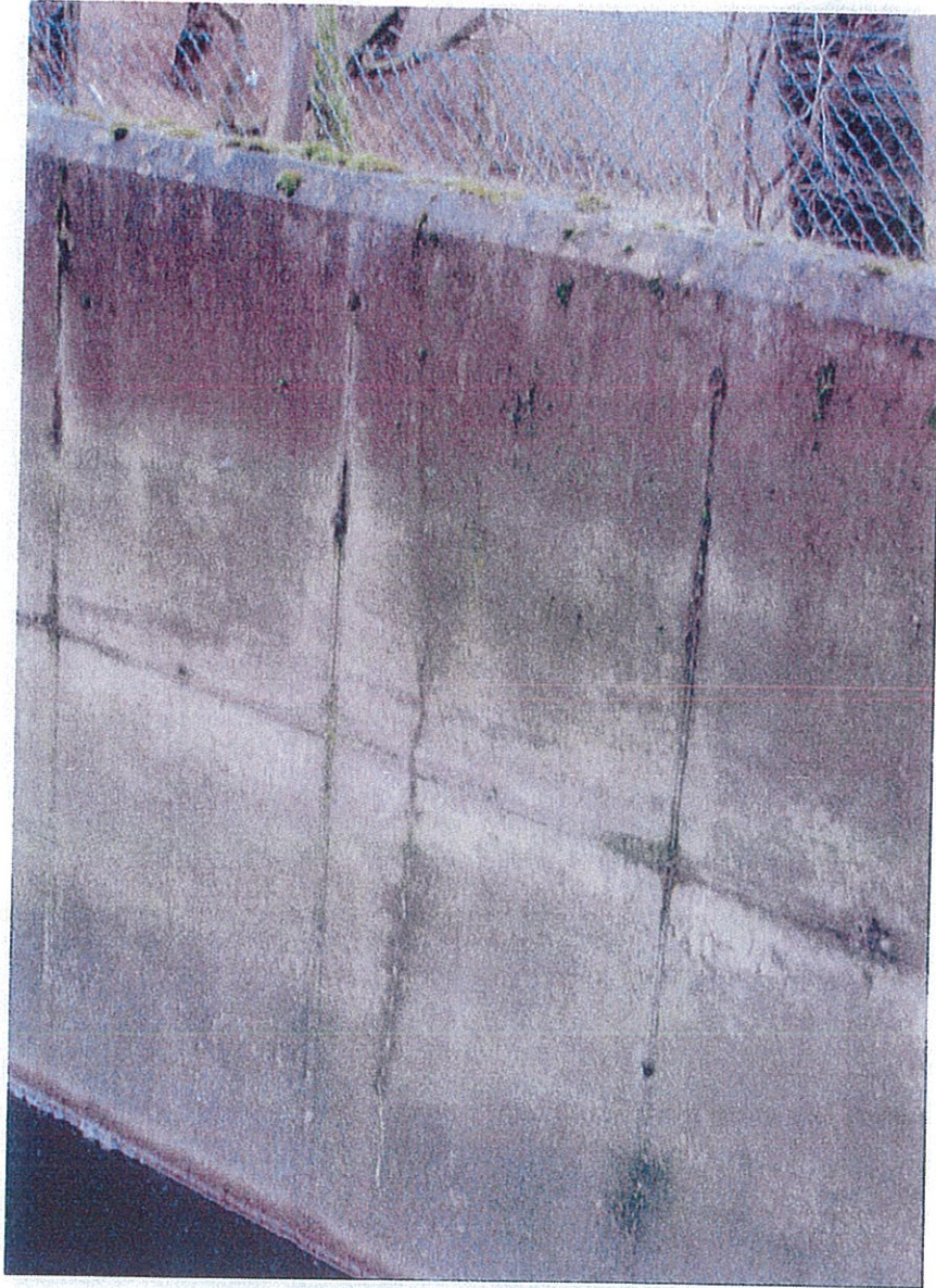
Photograph 6: South wall – crack on internal face
