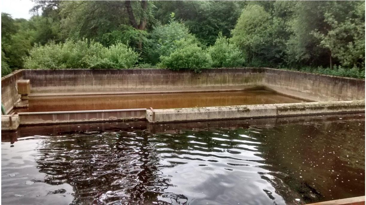
Photograph 4 – Leachate lagoon tanks
