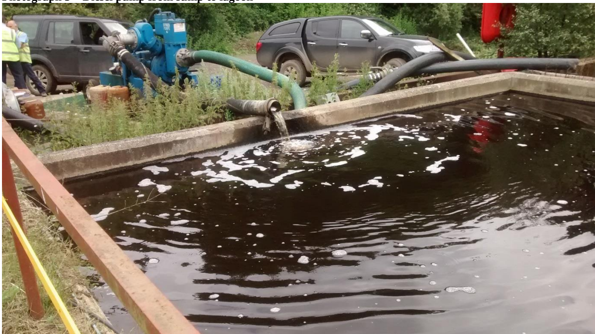
Photograph 3 – Diesel pump from sump to lagoon
