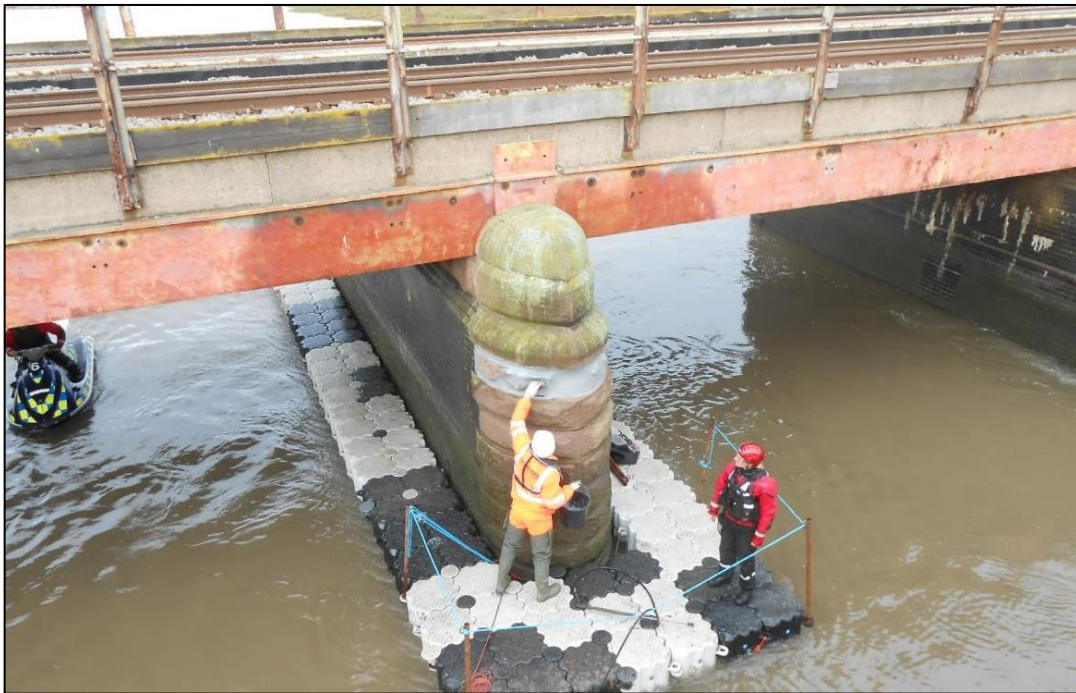
Figure 9: Example of pontoon wrapped around pier.
