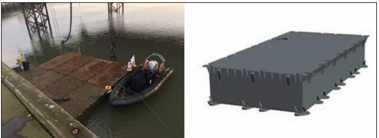
Figure 14: Example of metal pontoon platforms.
