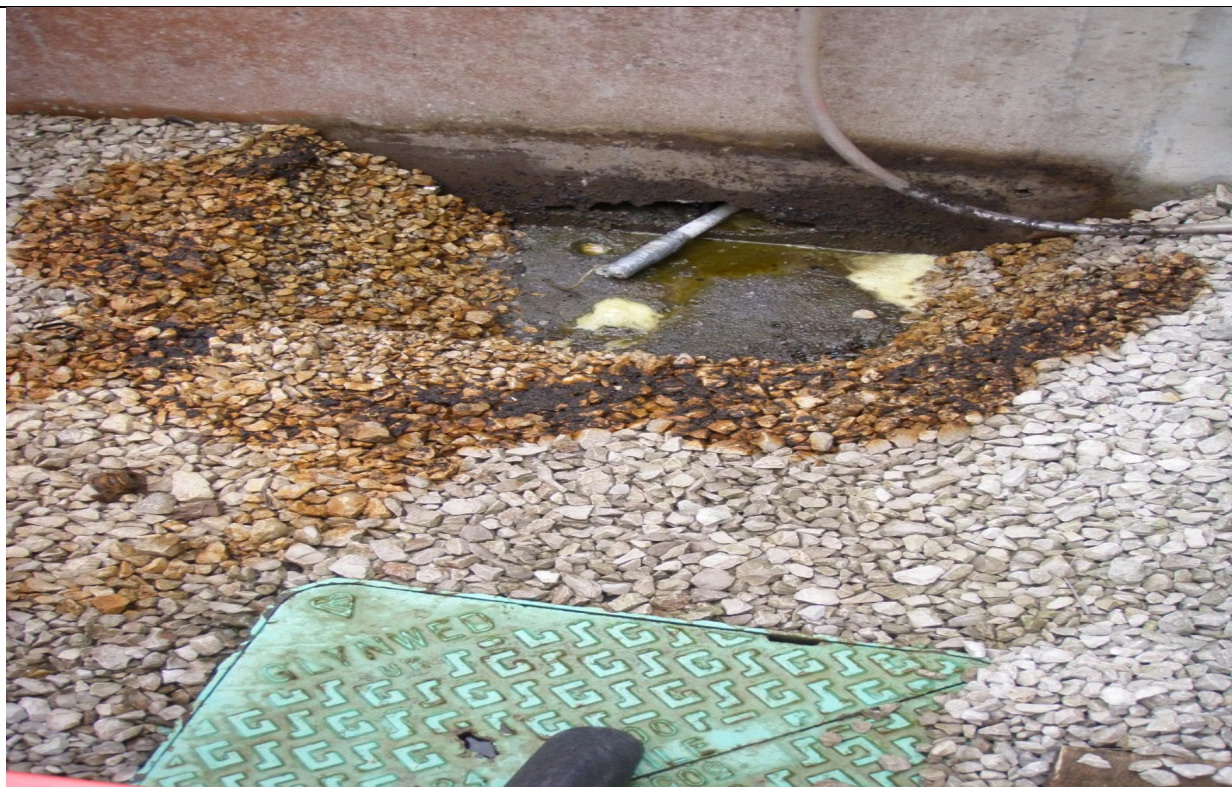
Damage to the outside of the bund
