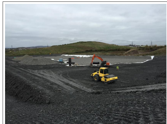
leachate stack to background, final clay compaction to area at foot of access ramp.
