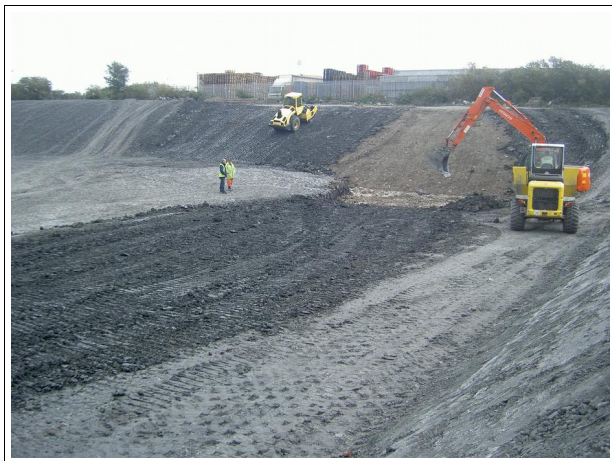
access ramp removed, E5 (foreground) regraded to accept overlapping repair along previous travel way, and F5 / G5 (background) excavated to subgrade in readiness for clay
