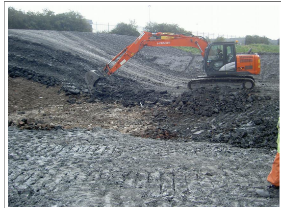
excavating access ramp (benching detail at neighbouring cell visible to left of photo)
