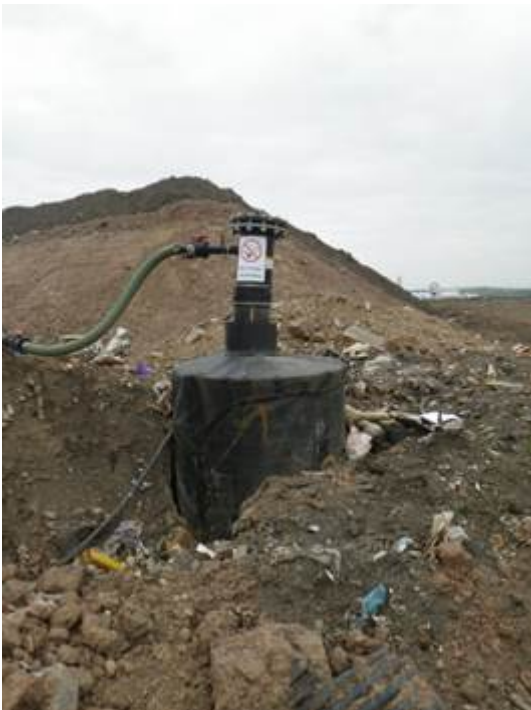
Photo 1: No smoking sign on leachate well
