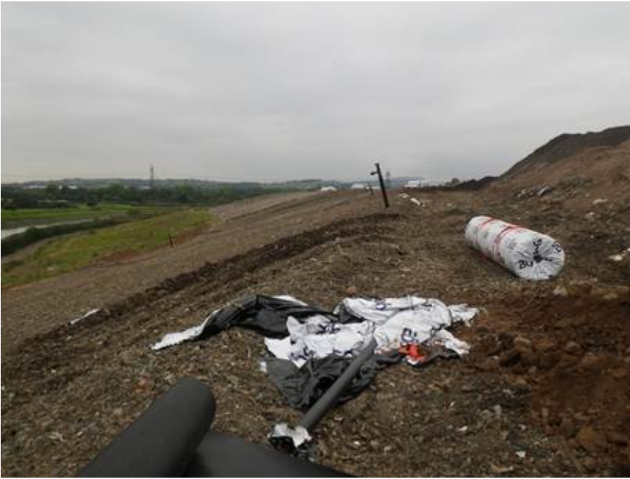
Photo 3: View west along flank to be capped over the laid regulation layer
