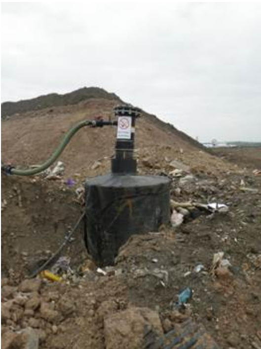
Photo 1: No smoking sign on leachate well
