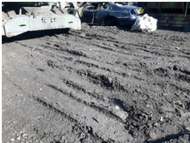
Photo One - Rutting of hardstanding surface
