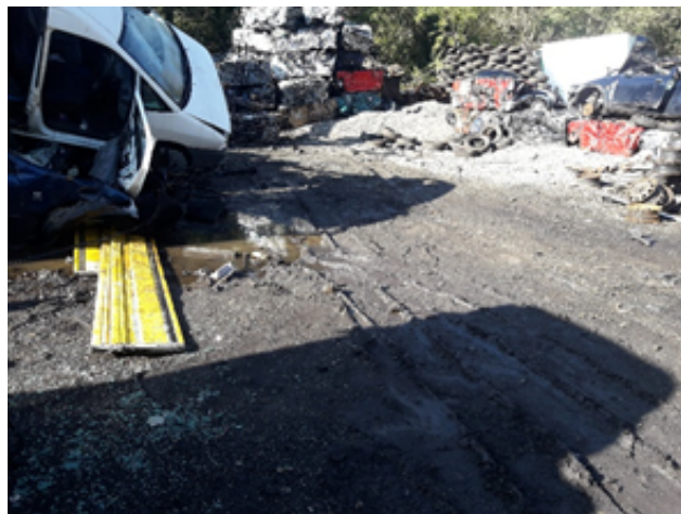
Photo Two - Rutting of hardstanding surface
