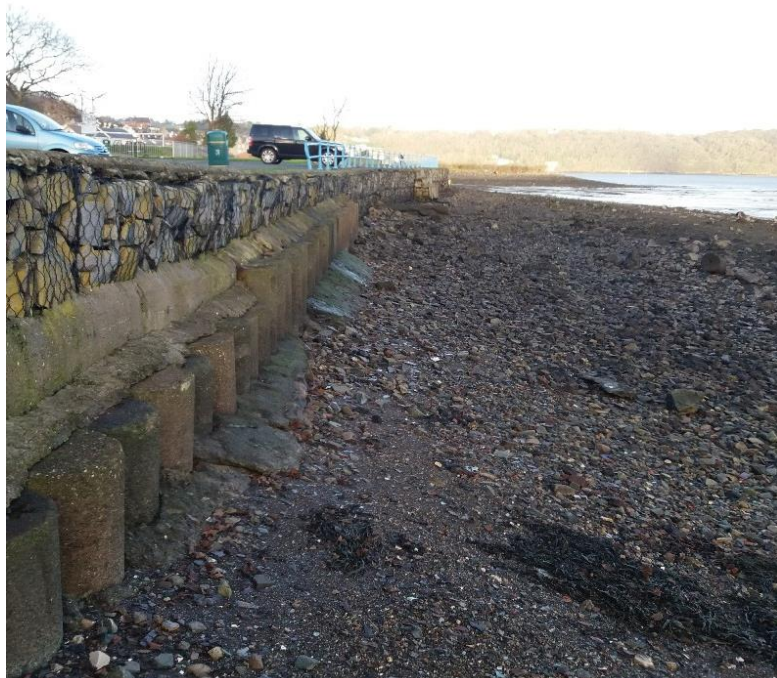
Photograph 6. View of existing sea wall and upper shore adjacent to the east end carpark.
