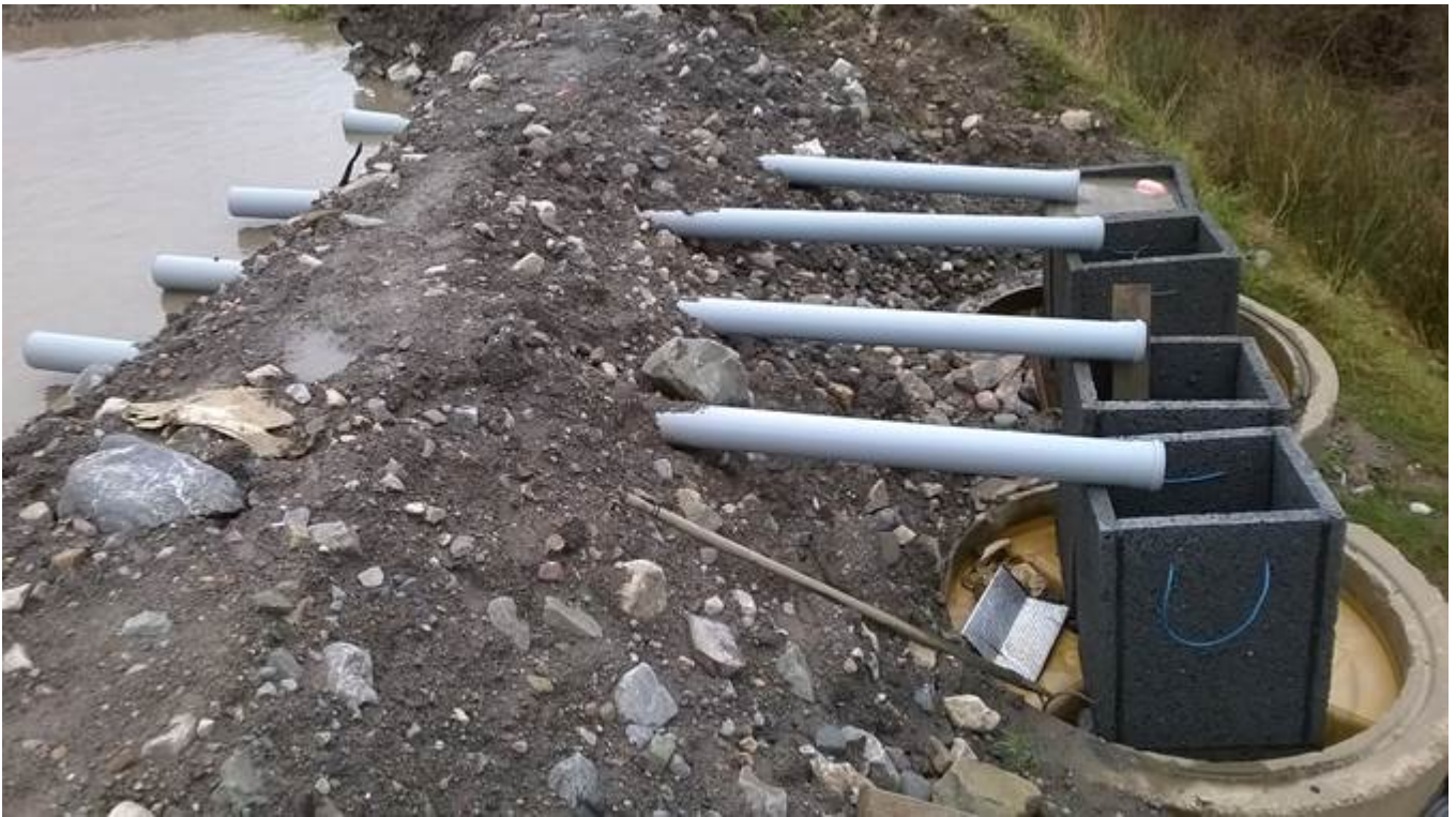
Photo 4 showing outfall pipes to the Hydroblox, with only the far block in use. The bund headwall construction requires immediate improvement so all four outfall pipes are providing an even flow.
