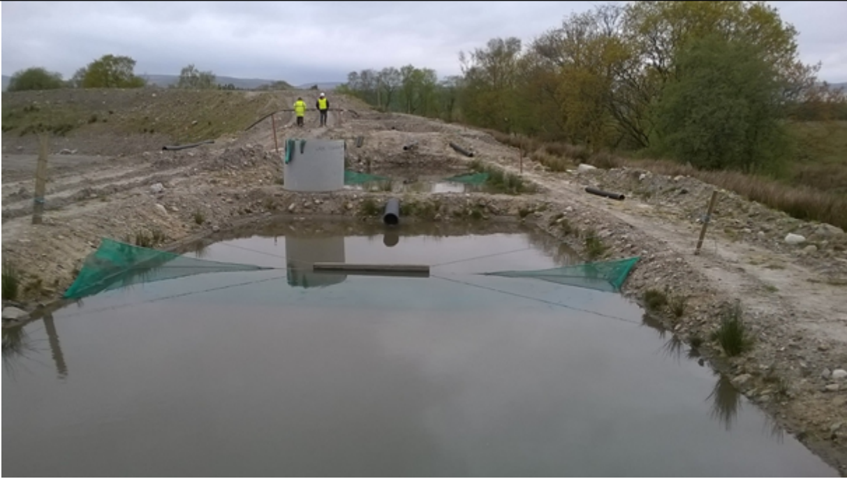
Photo 2 showing pipe positions between holding and settlement lagoons.
