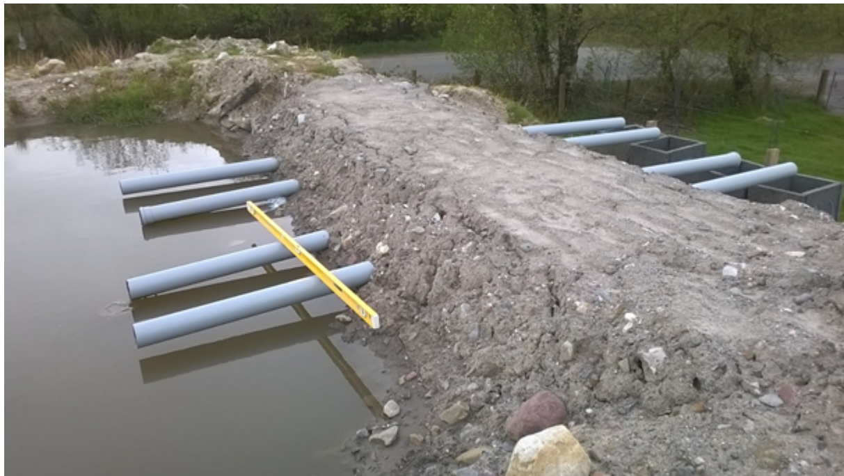
Photo 1 showing outfall pipes to the Hydrobox, which are not level. This design requires improving so that all four outfall pipes are stable, and can provide an even flow.
