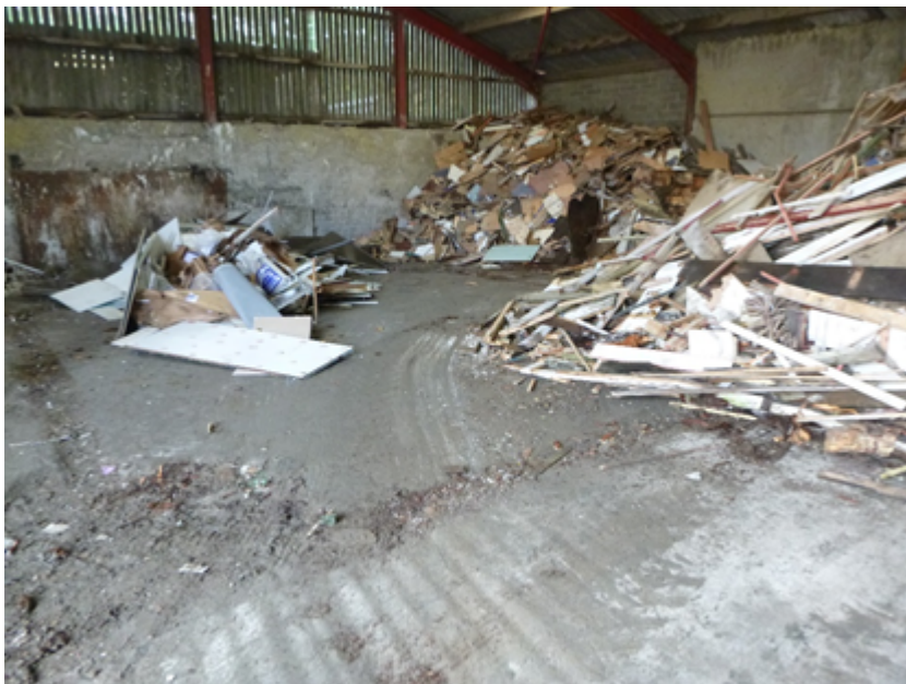
Photo 2. Looking into the main building, damaged concrete bottom left.
