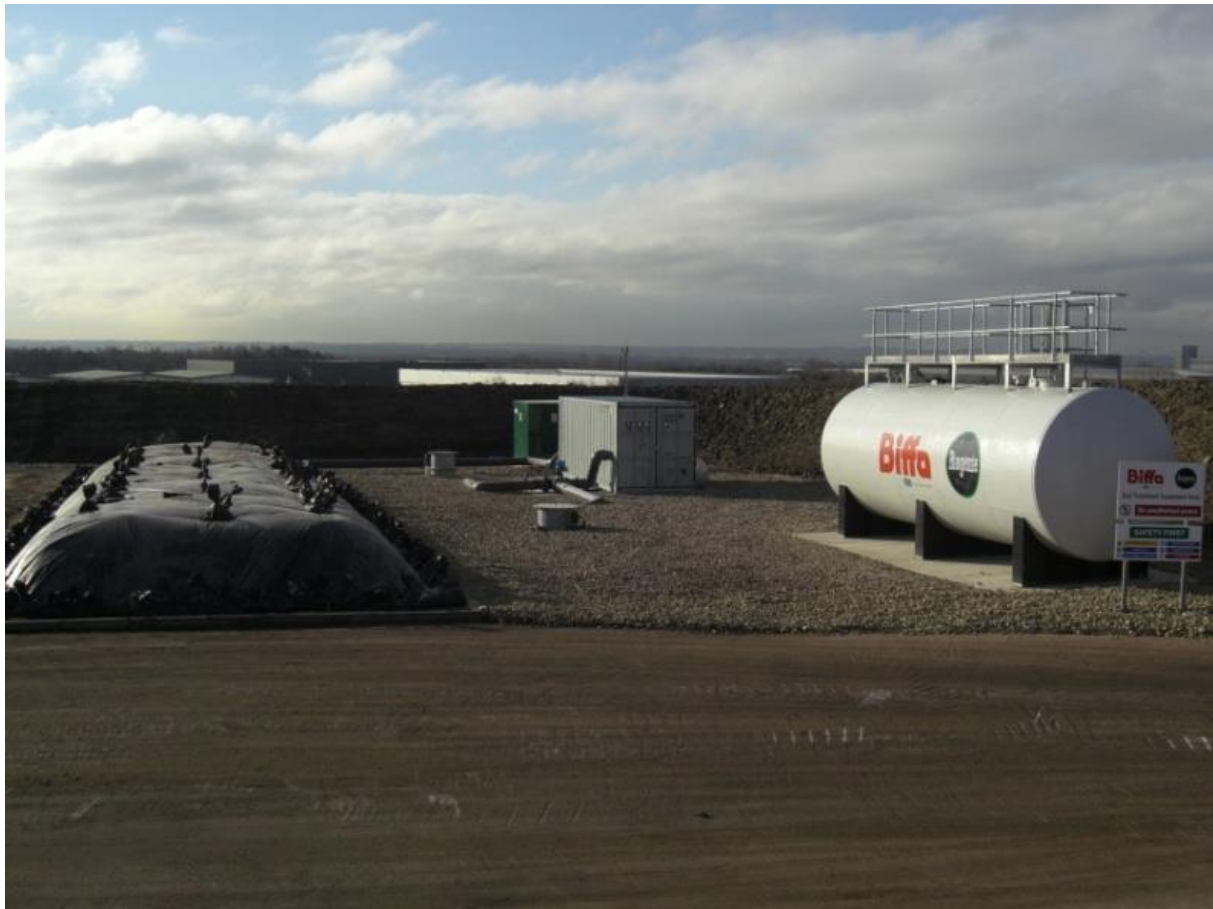
Figure 3-4 Biofilter and Process Water Tank
