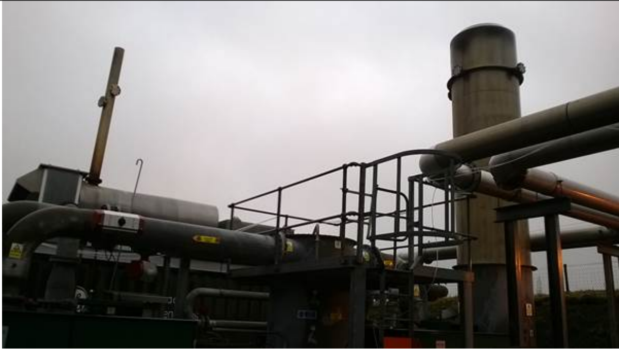
Overview of gas compound showing large flare stack on right and a jenbacher landfill gas engine on left.
