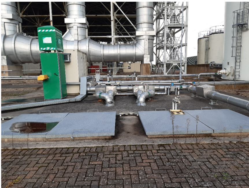
Photo 4. View of the neutralisation pit which accepts effluent from the water treatment plant
