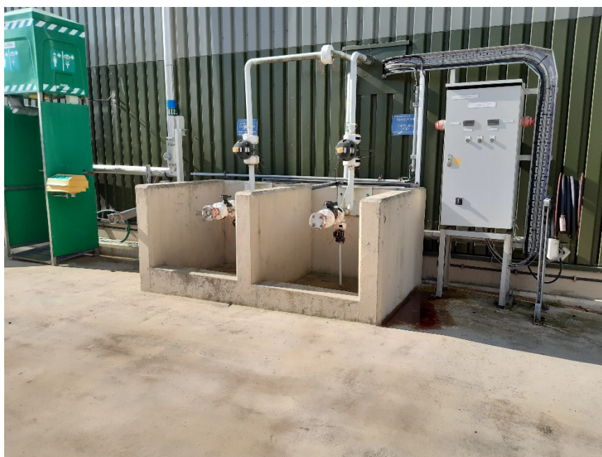
Photo 2. Fill points for the internal sulphuric acid and caustic soda tanks
