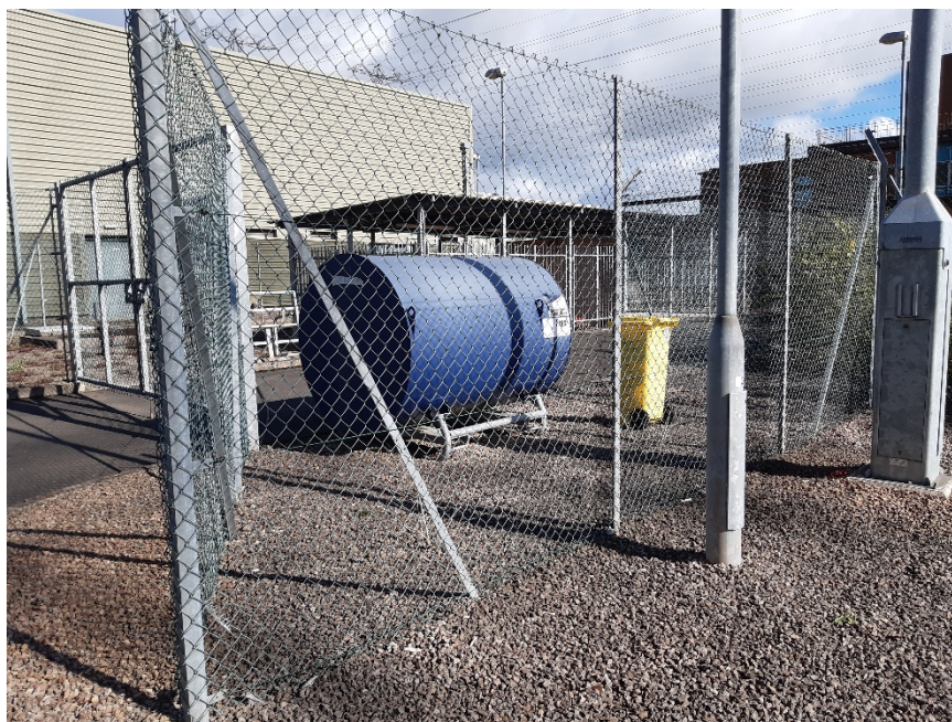
Photo 10. Double skinned diesel tank used for refuelling plant
