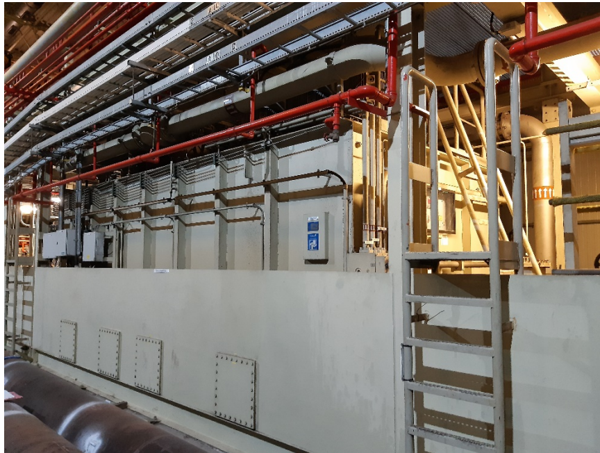
Photo 7. Lubrication oil tank located inside a bund which provides oil for the steam turbine system
