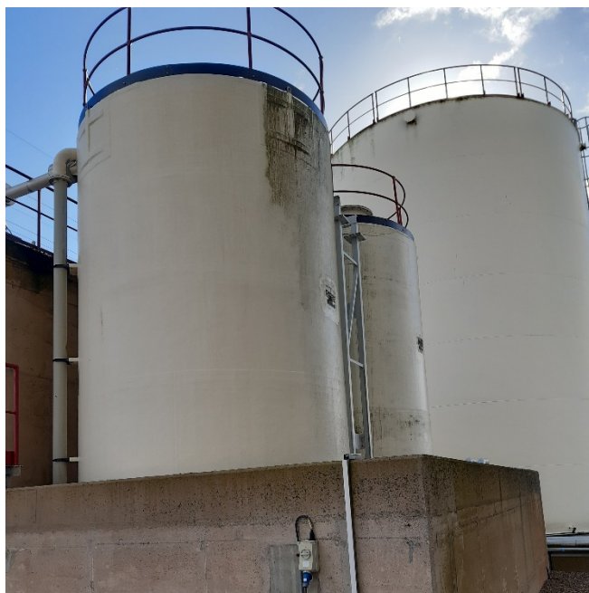
Photo 1. Two ammoniated effluent storage tanks. Water holding tank in the background.
