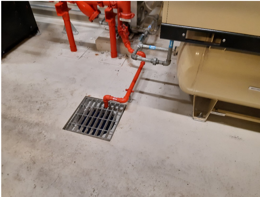
Photo 3. Example of floor sump inside of the water treatment plant
