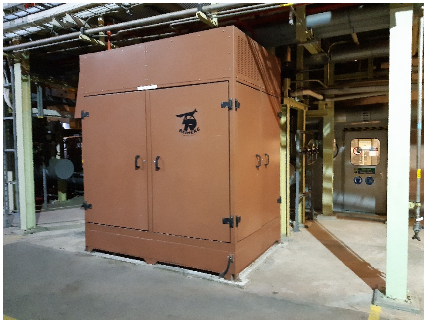
Photo 8. Hydraulic oil tank location
