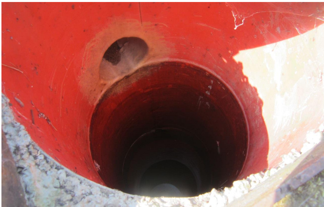
Photograph 6: TD2 following removal of the standing water. The water reached the level indicated on the wall of the chamber by the black coloured residue. The inlet pipe from the toe drain is observed towards the top photograph. No outlet pipe is visible from the ground surface.
