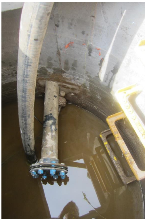
Photograph 3: TD1 pipework showing the fitted blanking plate. This is fitted to stop and potential flows between S1 and TD1.
