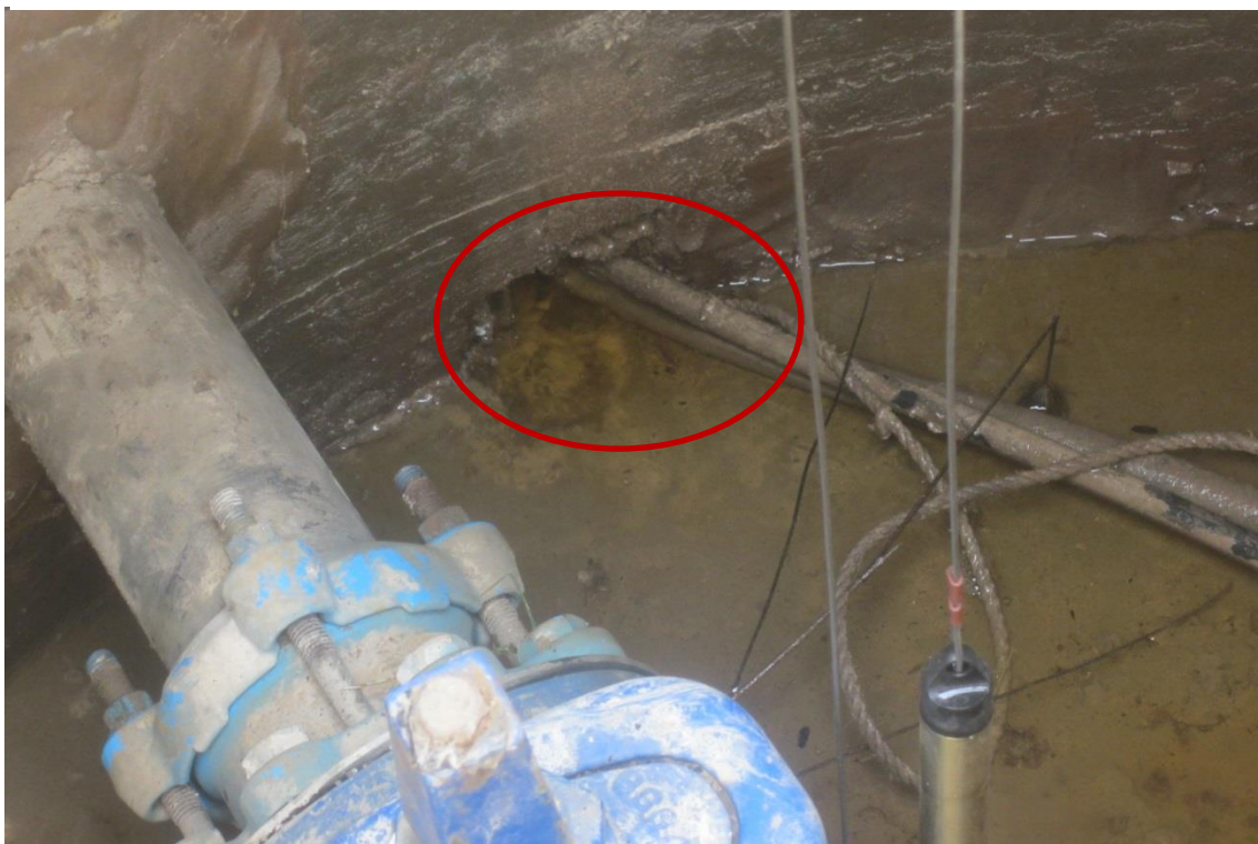
Photograph 4: Area of inflow into TD1. Several cables enter TD1 through the concrete (see the red circle), and it is this area that leaks water into TD1.
