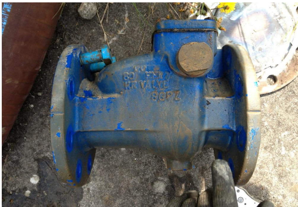
Photograph 2: Non-return valve after removal from TD1 pipework. It was installed in a direction where flow was stopped from the toe drain and allowed from S1 to TD1.
