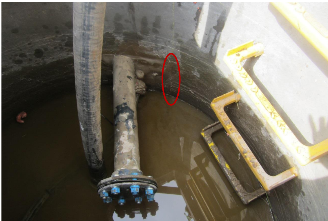
Photograph 5: Area of inflow into TD1. A vertical seam in the concrete ring chamber casing (see the red circle) appears to be poorly sealed and allows water to leak into TD1.
