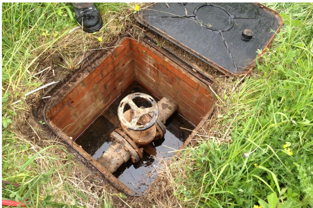
Photograph 8: Emergency outflow pipe and valve from TD2. TD2 is located towards the bottom left of this photograph.
