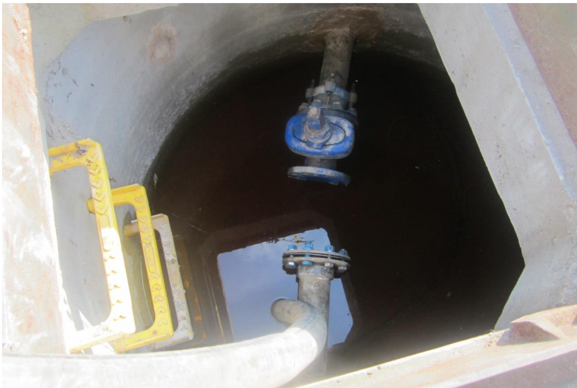
Photograph 1: TD1 drain chamber with the non-return valve removed and the blanking plate fitted. The pipe at the top comes from the toe drain, and the pipe at the bottom goes to the sump (S1). The temporary pumping pipe is also visible from the surface.
