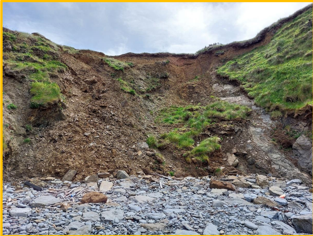
Figure 35 View from beach of eroding cliff at location of promontory port (MSDS_Erebus_073)
