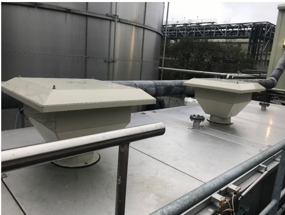
Figure A2.2: Carbon Odour Control Unit on DAF Outlet
