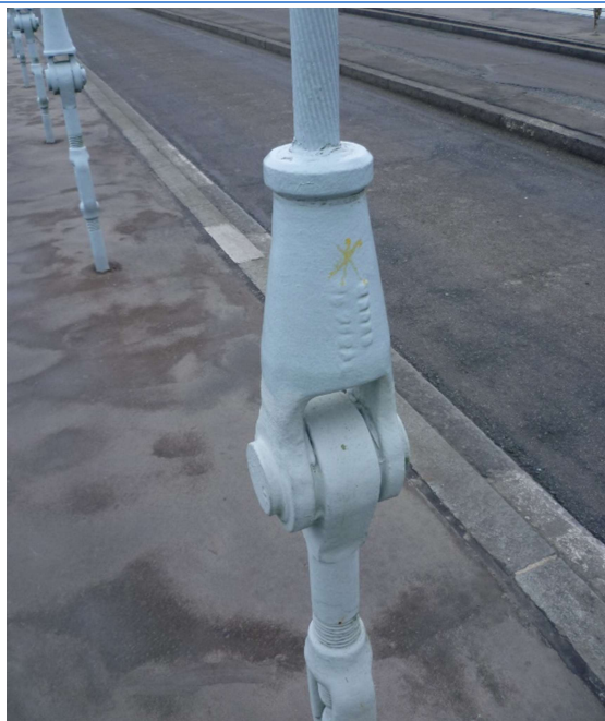
a) Drop-link and turn buckle on the base of the supporting hangers.
