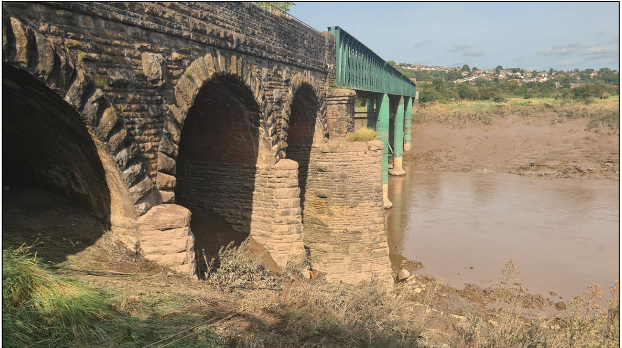
Figure 1: Embankment failure - June 2021.
