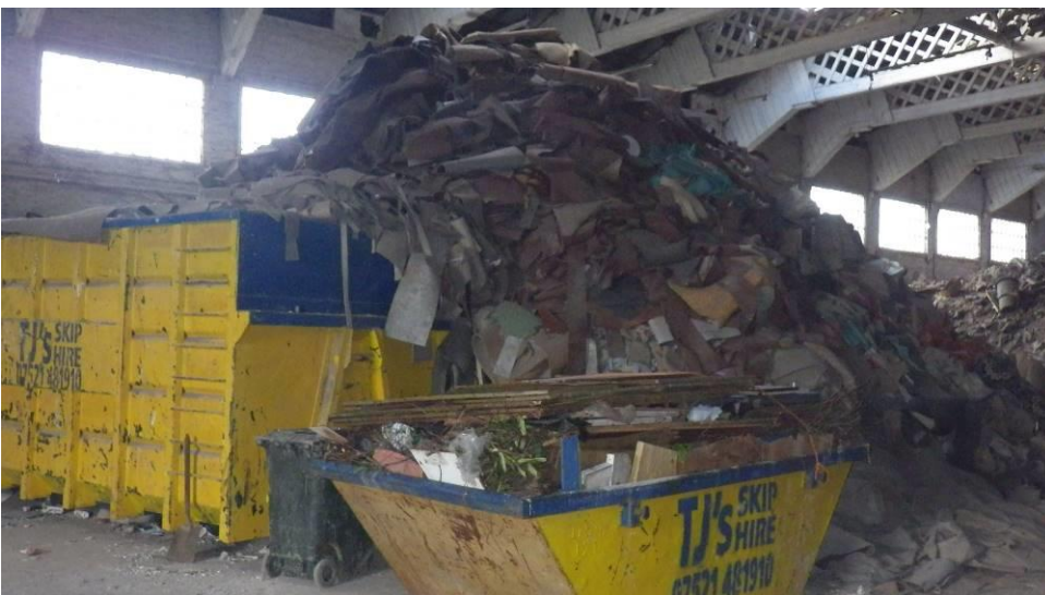
Substantial amount of carpet waste on site
