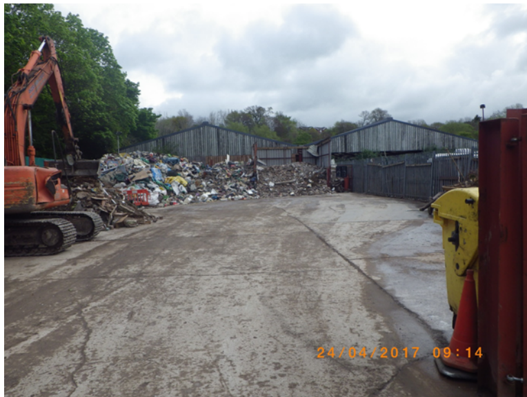
Waste piles on site (24/04/2017)
