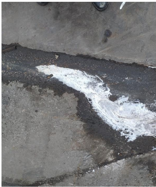
Spills in area of concrete jointing/ cracking adjacent to the tank farm
