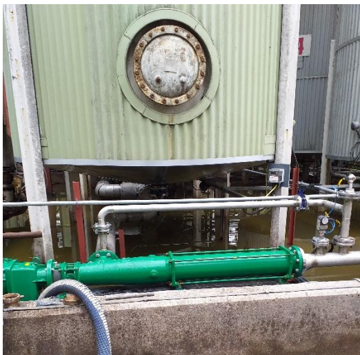
TS tank farm bund approx. 1/3 rd full of rainwater
