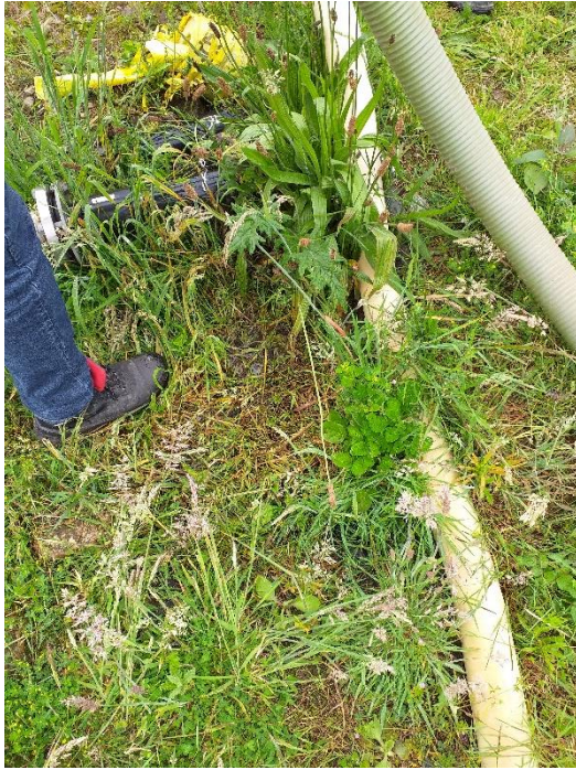
Ground below dripping lagoon pipework manifold
