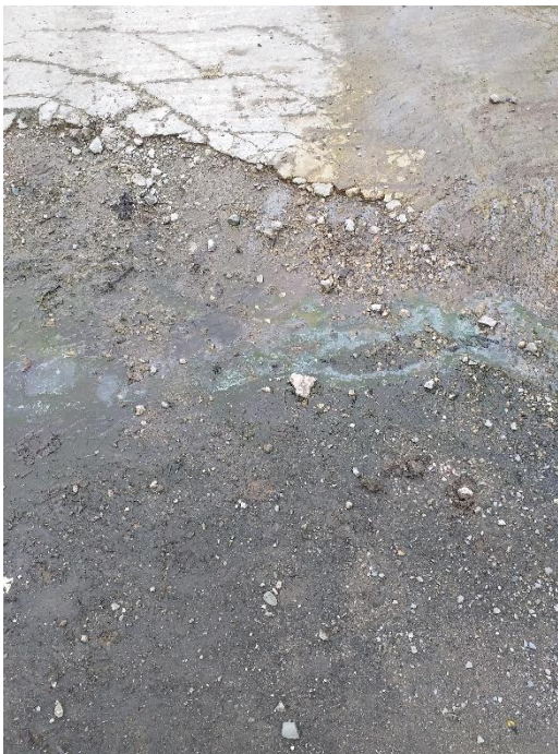
Concrete degraded on lower yard area adjacent to lagoon access ramp
