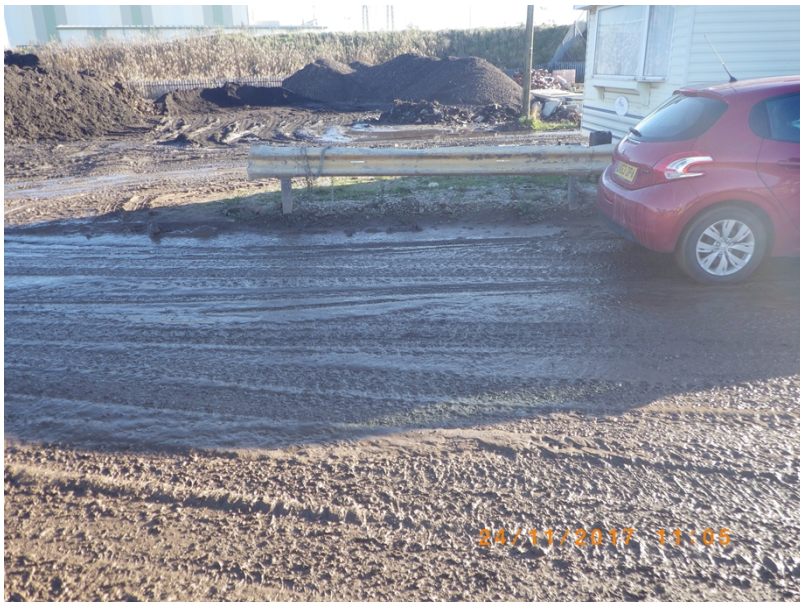
Mud on tracks around site
