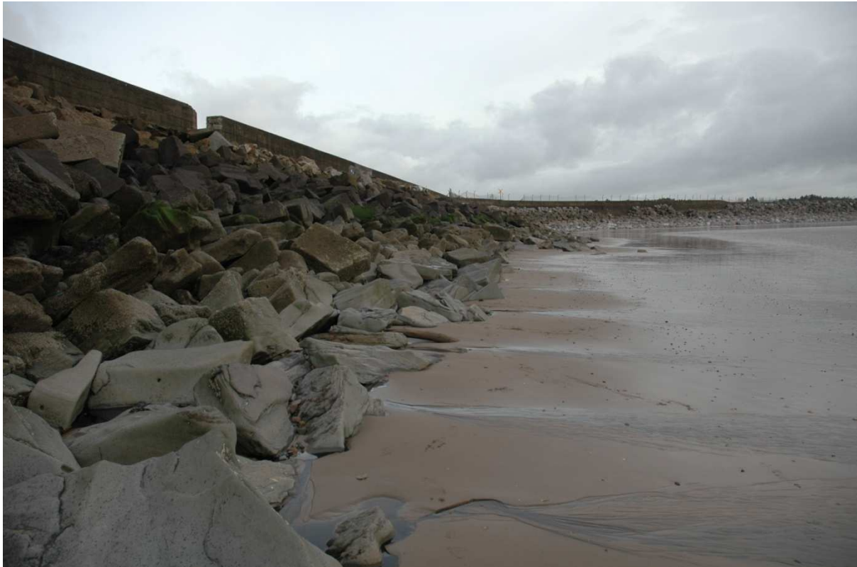
Photograph 18.1 Port Seawall, adjacent to the former Queen's Dock Oil Terminal, looking eastwards towards the former tank farm area. Note groundwater seepages from base of Port Seawall. Site Walkover Survey, 7 February 2013.
