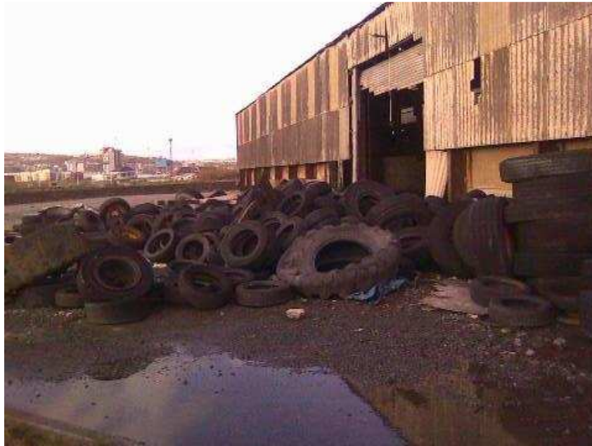
Photograph 18.4 Derelict building at the western end of Area A. Note the condition of cladding and fly tipped tyres. Fragments of cladding and other burnt and discarded wastes are visible on the ground surface (7 February 2013).
