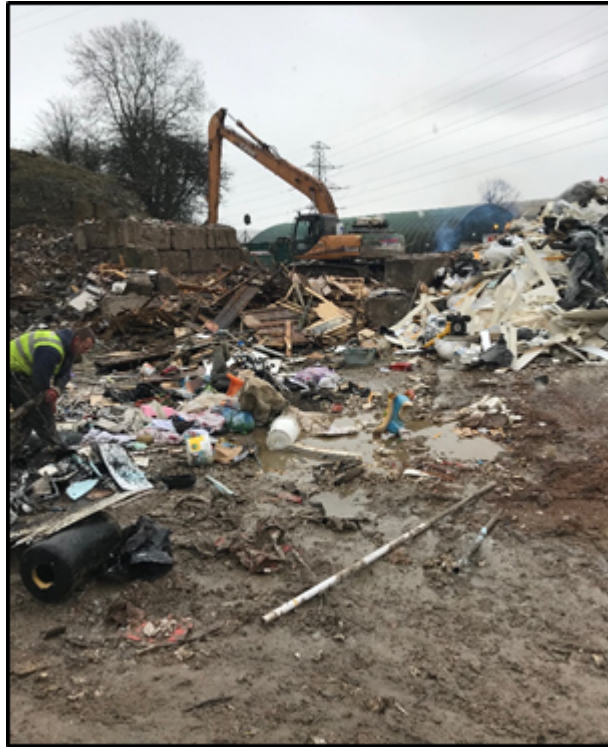
Picture 2 – showing infrastructure in need of repair in the upper yard.
