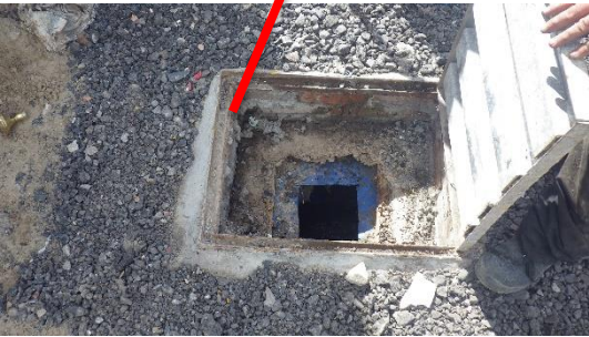
Sump for sealed drainage
