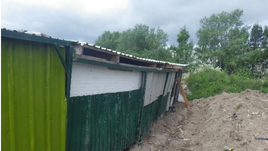
Areas of rear of building requiring repair
