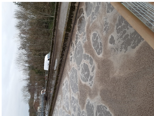
Photo 4: Aeration lane 1, Zone 2 not aerating.
