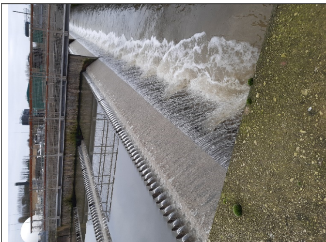
Photo 3: Weir at PSTs – Flow heading to aeration lanes.
