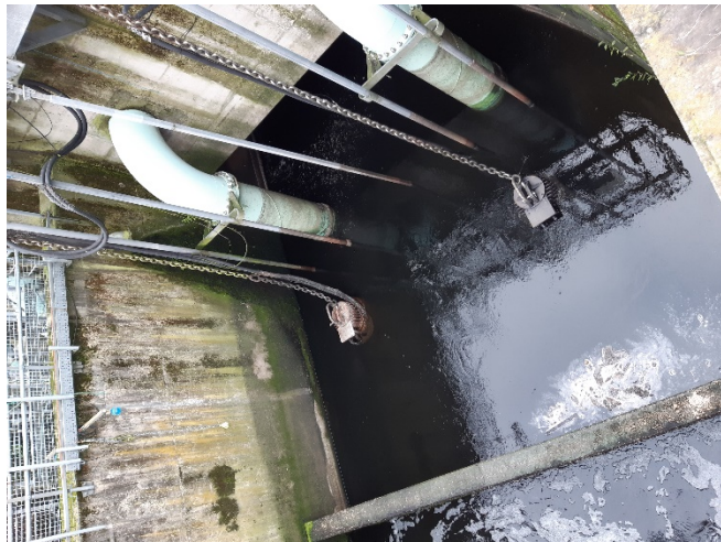
Photo 7: Well containing FE before discharge to Lavernock Point.
