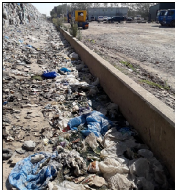
Photograph 9 | taken on 15/07/19 - showing residual waste material in the Field 1 drainage channel
