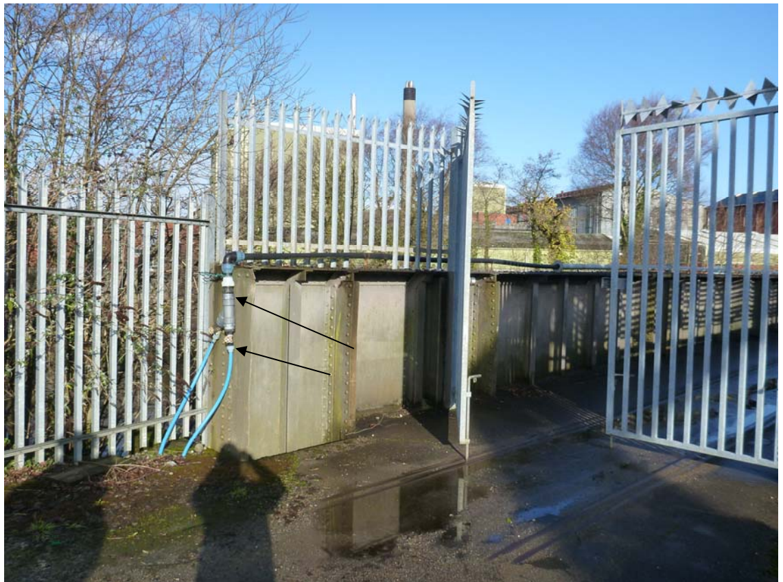
Photograph showing leachate transmission pipework over the access bridge crossing the main river. The fixtures are screwfix type.
