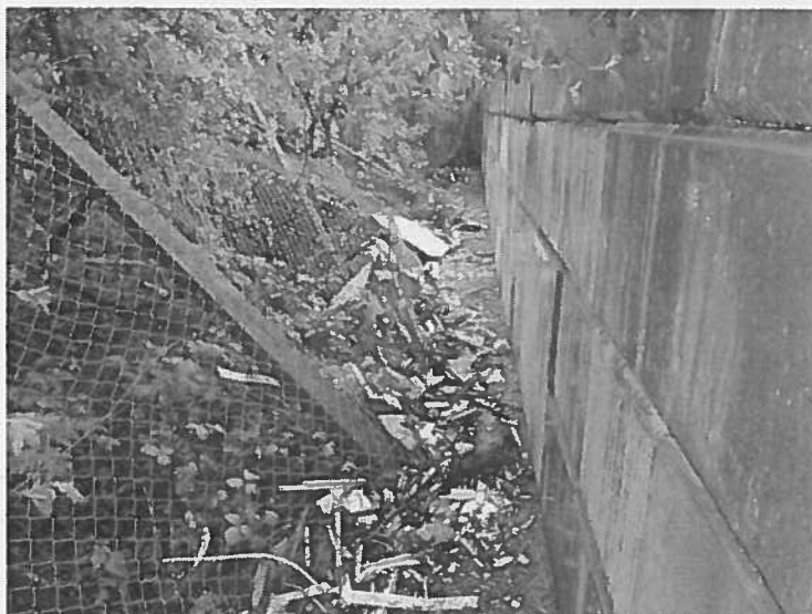
Photo 5: Caution must be exercised when loading & unloading from the push wall bays to ensure that the product does not overspill into the areas between the bays and perimeter fencing
