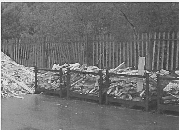
Photo 4: Despite previous concerns the site security fencing was in a particularly poor condition
