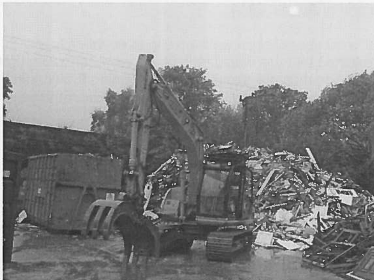
Photo 3: Waste pile being removed during the visit
