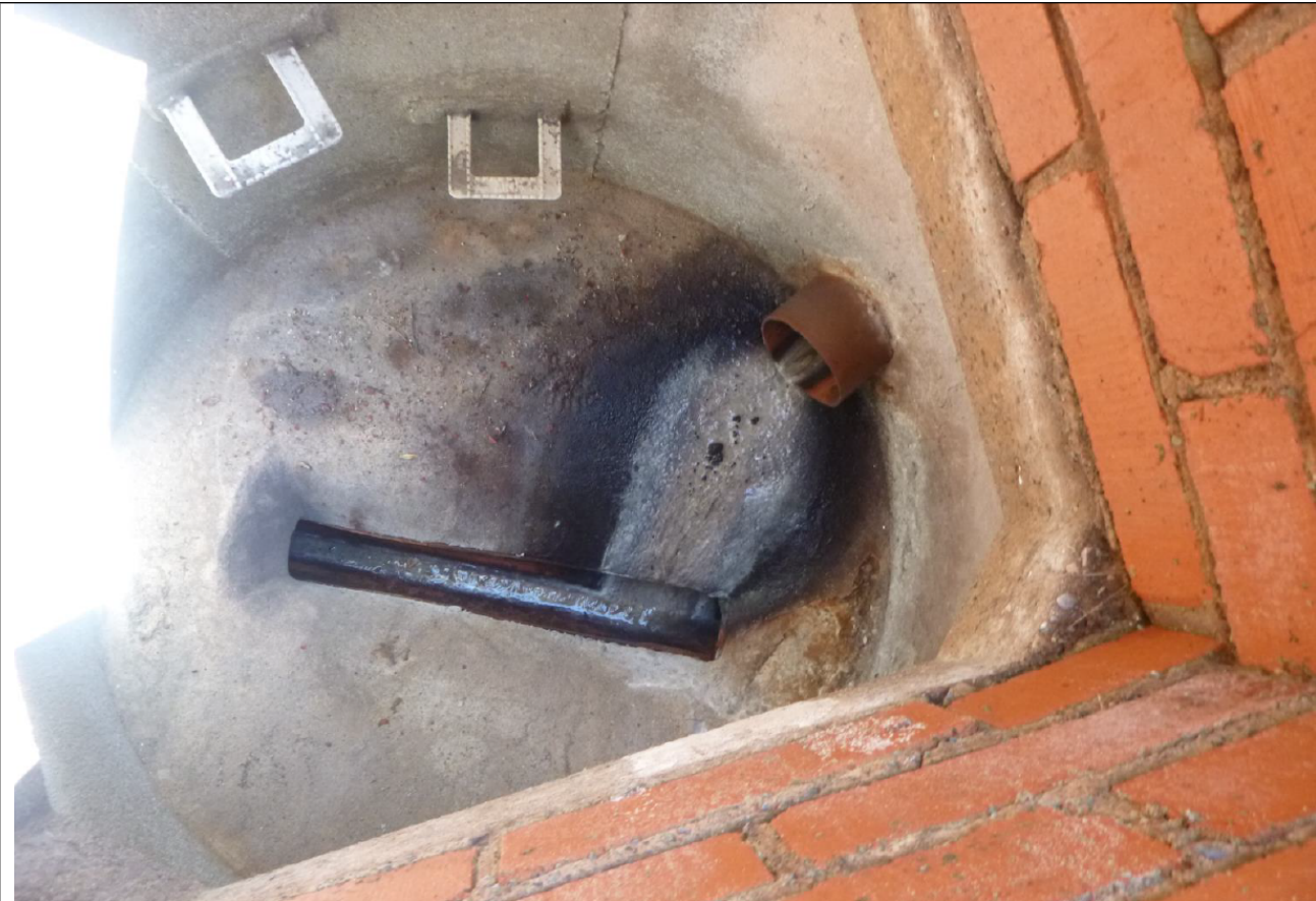
Photograph 2: Final Effluent sample chamber.
