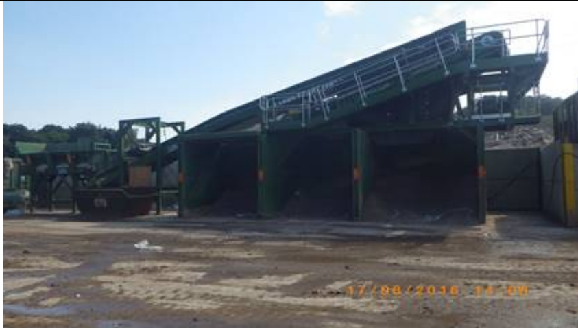
Photo 1 – New waste treatment plant located near the new waste transfer building
