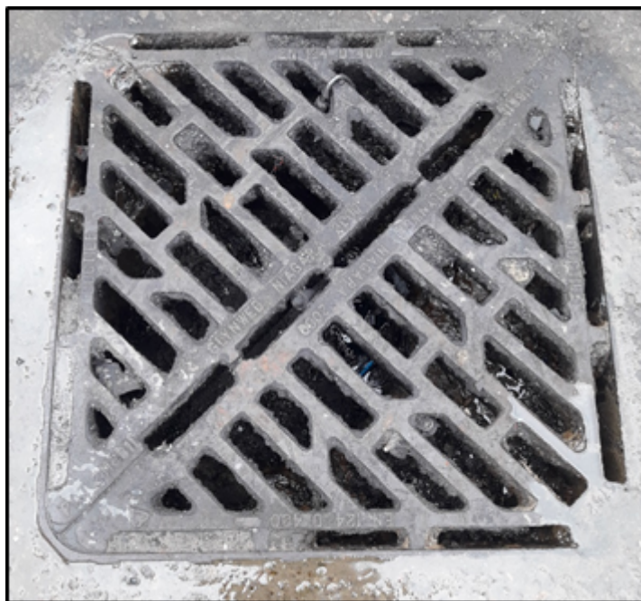
Picture 1 – showing the clogged drain in the yard on 19/03/19
