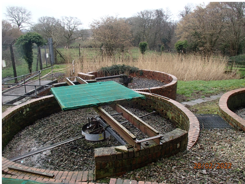
Photo 2 - filter bed, humus tank and reedbed
