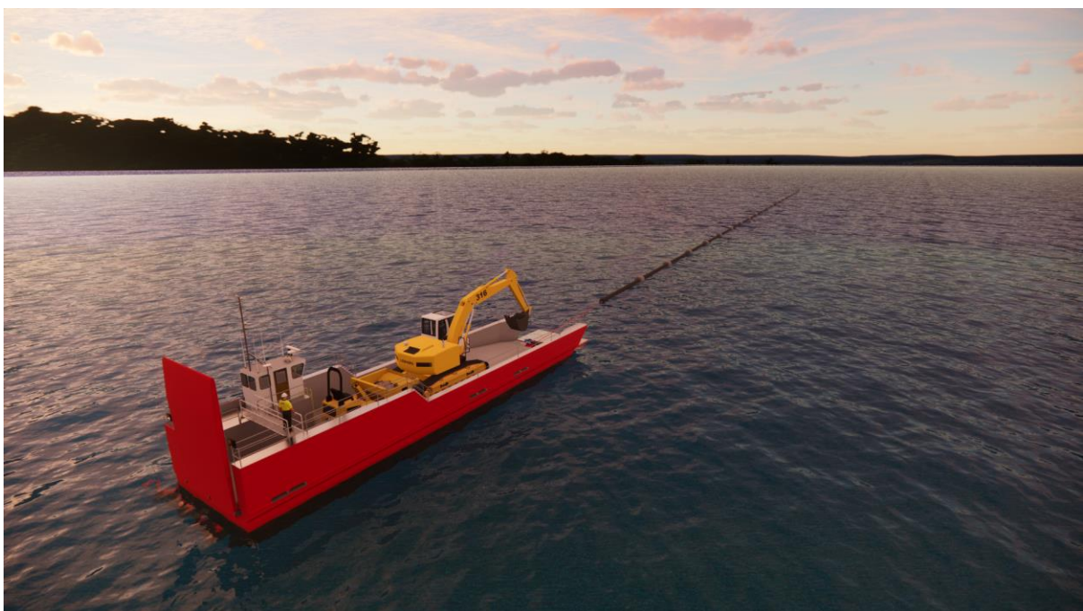
New pipe being transported from the harbour facility into the required position.
