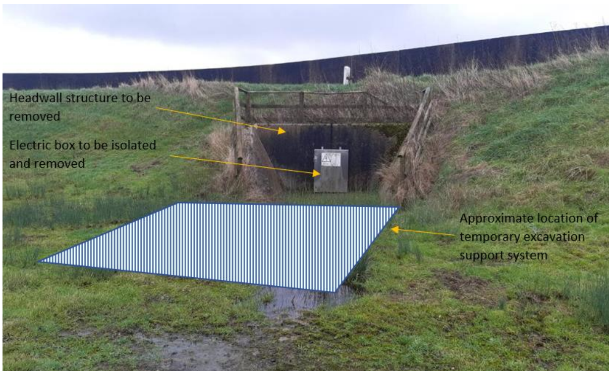
Photograph showing the electricity supply and surrounding structure
