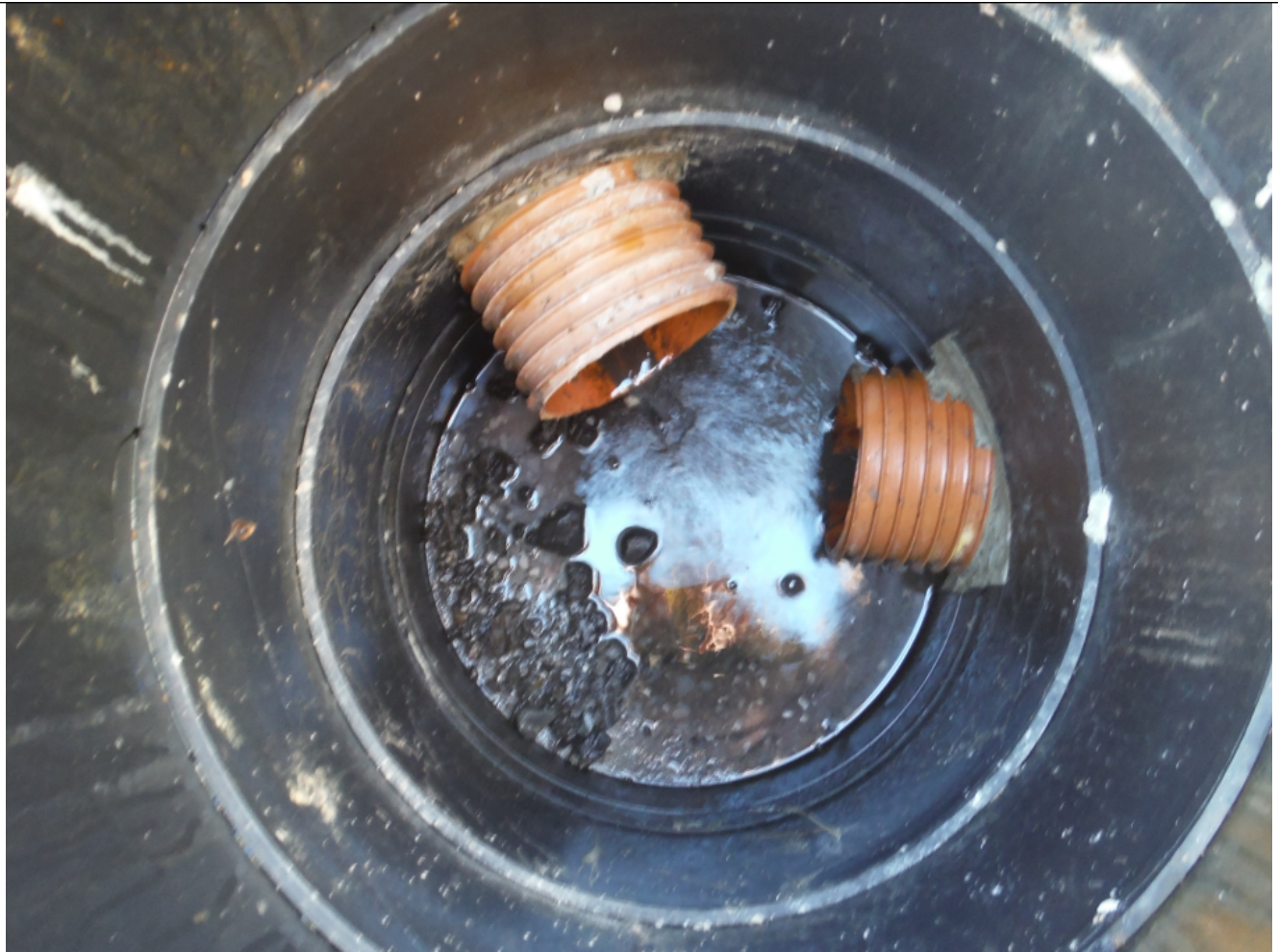
Photograph 2: Final Effluent sample chamber.
