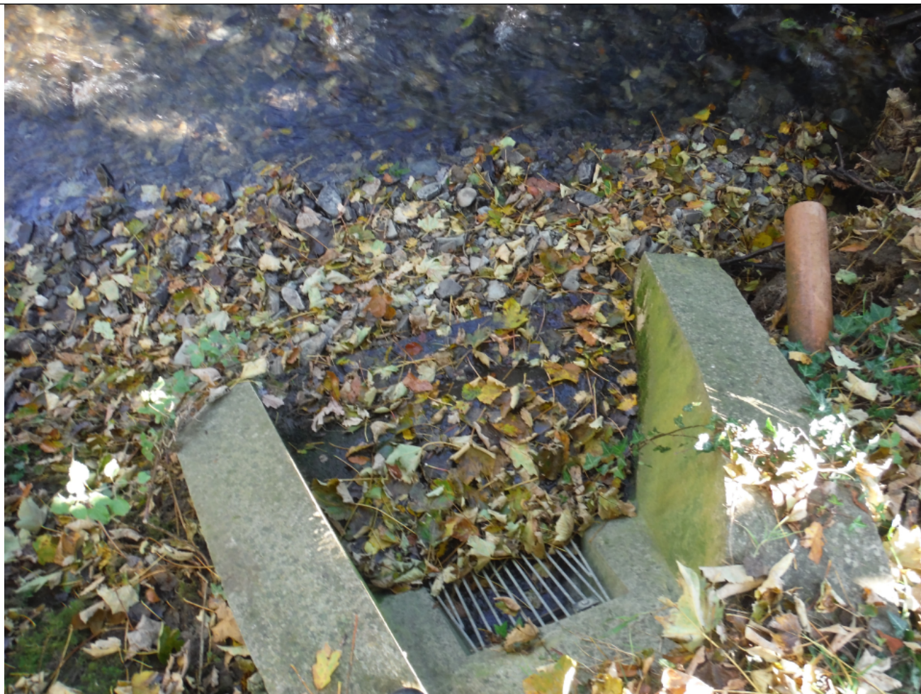
Photograph 3: Final Effluent discharge point headwall.
